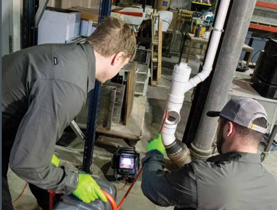
Colin Luttrell and Nick Iachetta use a RIDGID FlexShaft K9-204 machine to clear a drain.
