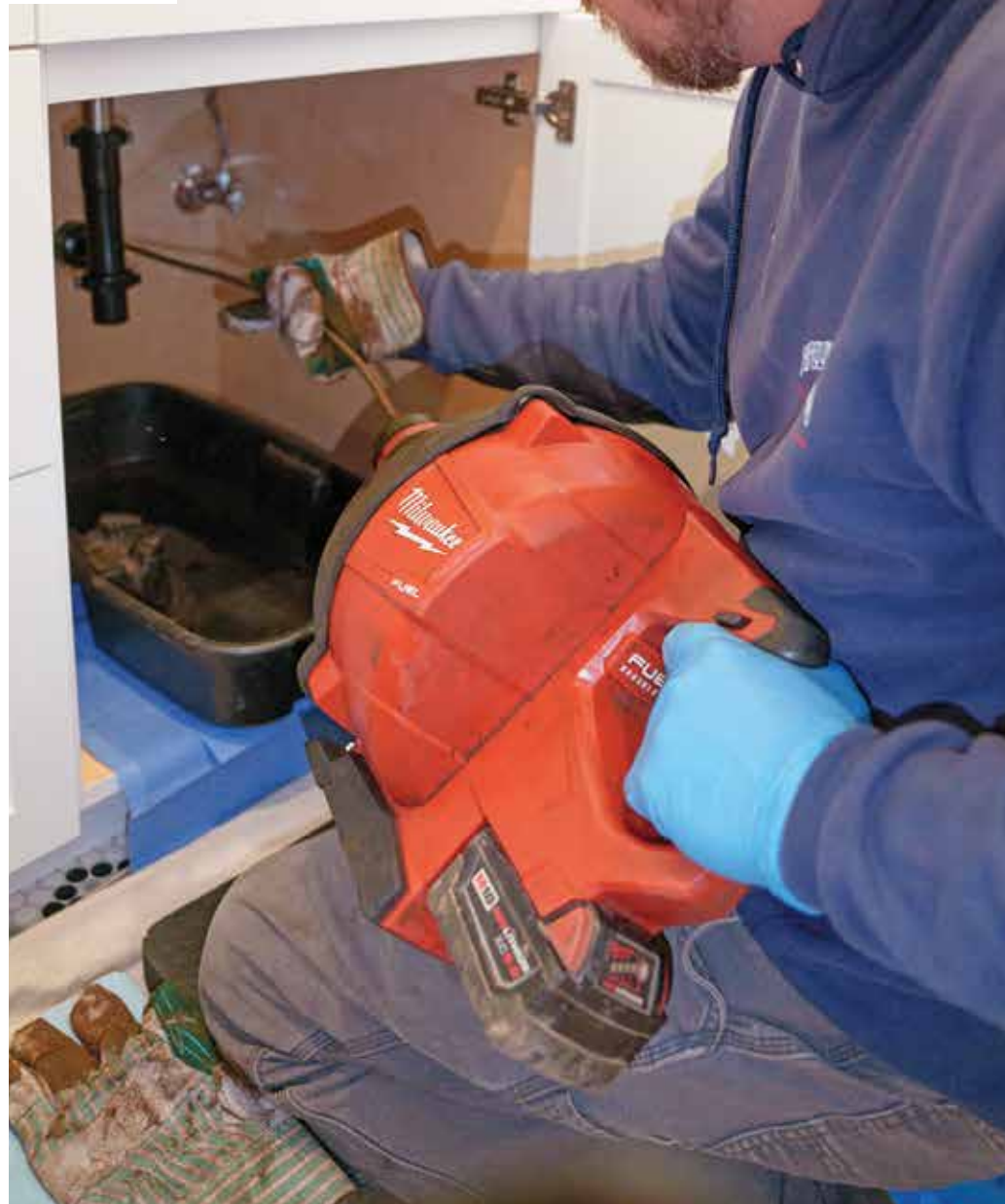
➤ Drain technician Brent Steele uses a Milwaukee M18 drain snake to clear a bathroom sink clog.
