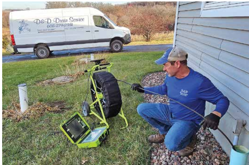
▲ Dan Kalschur, owner of D & D Drain Service in Lodi, Wisconsin, uses an Opticam push camera from Insight Vision to inspect a residential sewer line.
