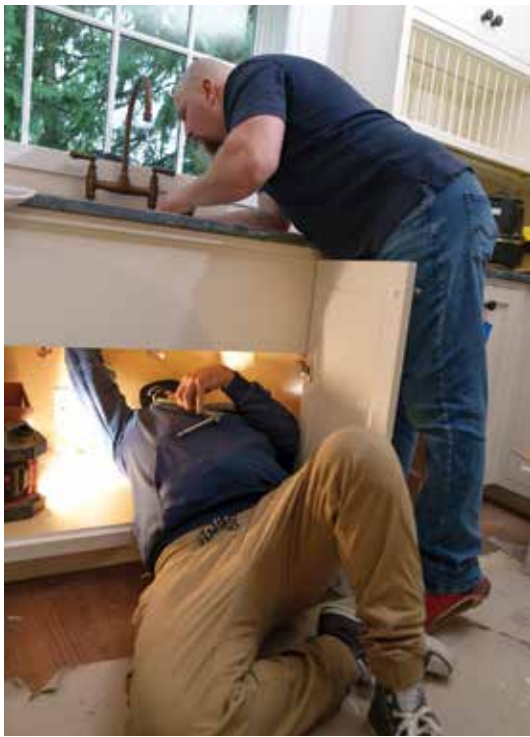
Apprentice Joshua Reyes and journeyman plumber Ken Galvin work on a kitchen remodel. Pipeline Plumbing maintains two categories of focus for plumbing crews — service plumbers and remodeling/new construction plumbers.
