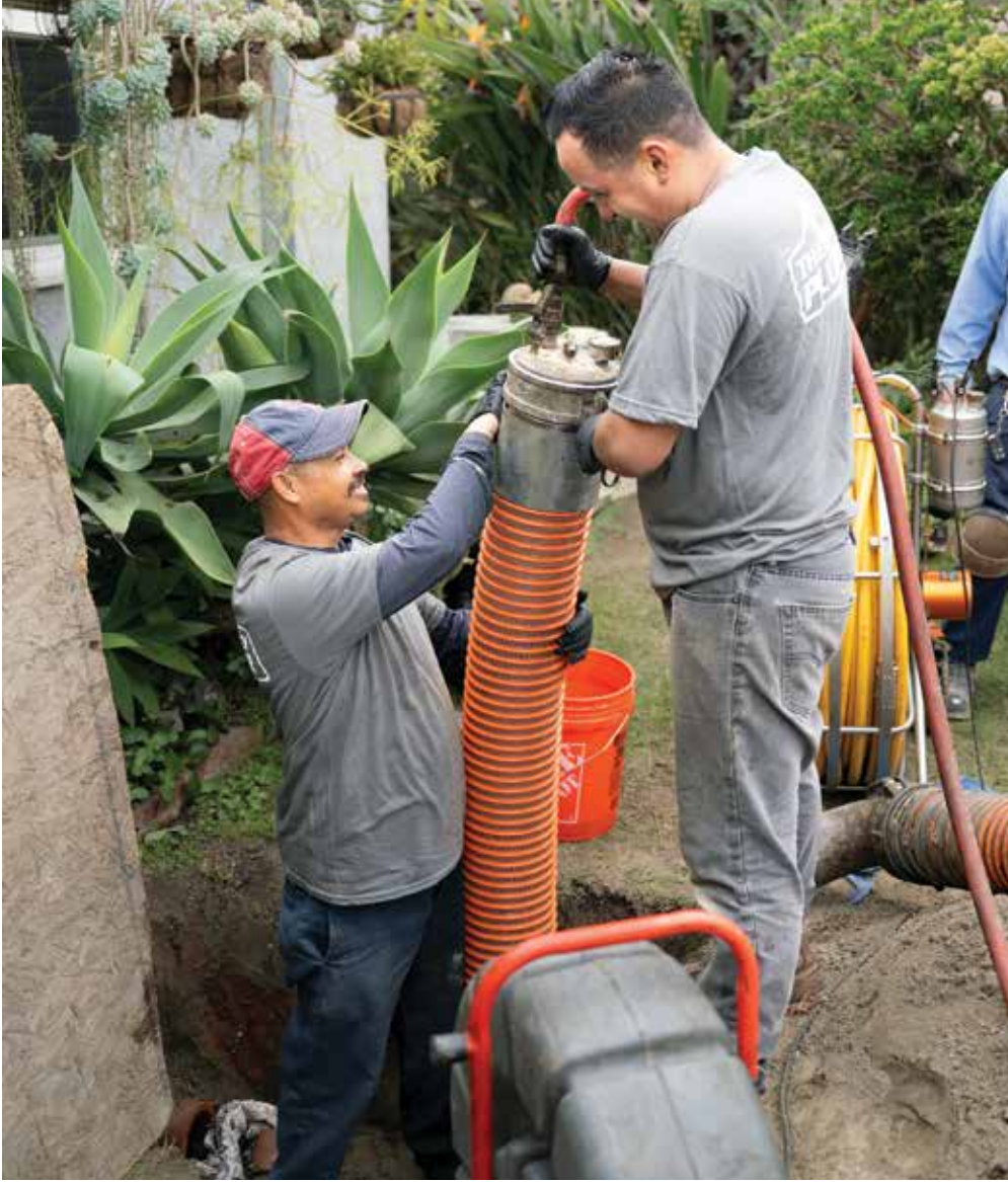
▲ Jesus Orantes and Juan Contreras inflate a liner. The Family Plumber uses pipe lining equipment from Perma-Liner Industries.
