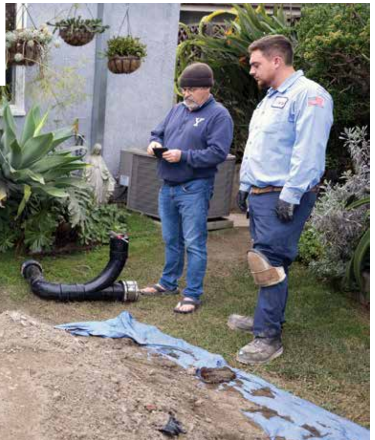
✔ Jesus Orantes prepares to send a RIDGID SeeSnake inspection camera down the line as homeowner Kristoff Przyucki and fellow technician Nick Ruiz look on.
