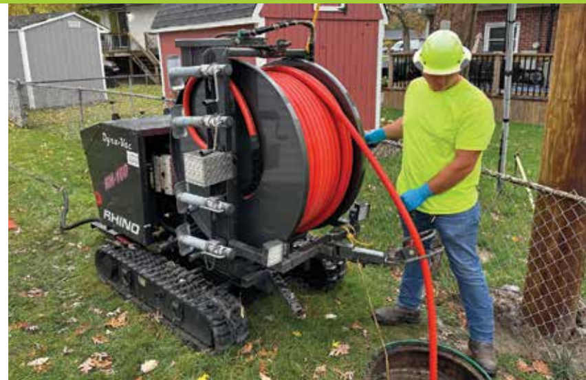
▲ Steven Bucklin, co-owner of Absolute Pipe, uses the Dyna-Vac Rhino RH-100 jetting machine. Pipe cleaning jobs with difficult access points haven’t been a problem since the company acquired the unit.
