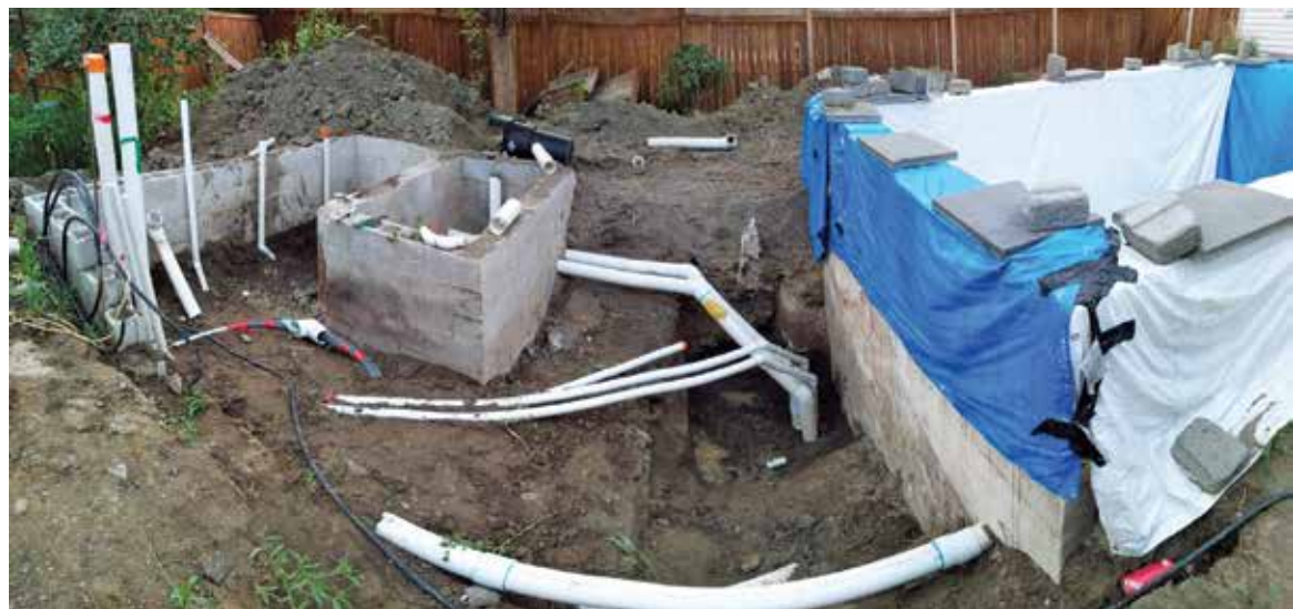
⚡ The best koi pond designers use a wide-diameter pipe, like 4-inch or larger, with no angle fittings. If corners need to be made, they should be 90-degree sweeps or flex pipe. (Photos by James Careless)
