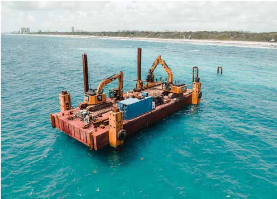
« Two Caterpillar excavators, a Cat 323 and a 336, operated by Earth View sit on a jack-up barge off the ocean coast near Boca Raton, Florida.
