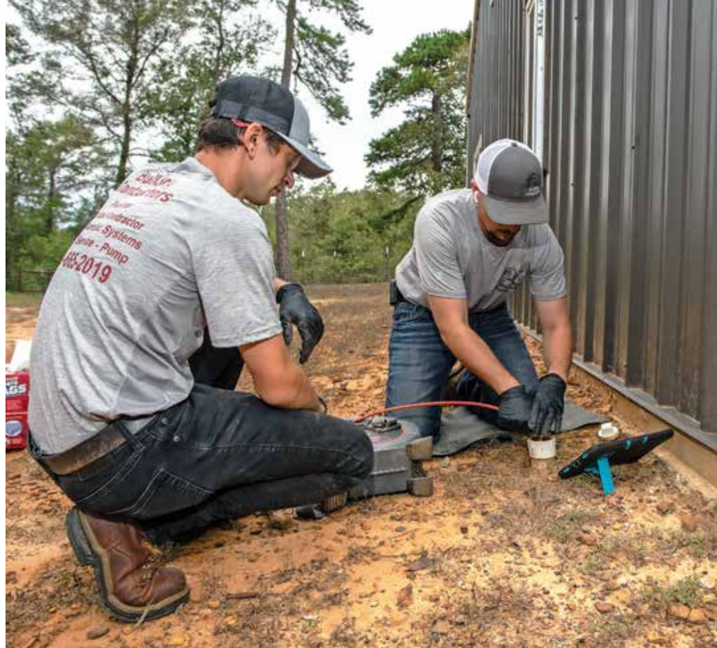
Nathan Harrah and Jeff Keller use a RIDGID FlexShaft drain machine. The company also uses drain cleaning equipment from General Pipe Cleaners and Milwaukee Tool.
