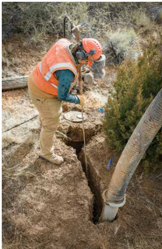
⚡ When exposing utilities, contractors should always keep their nozzle 8 inches away from the utility to prevent damage to both the equipment and utility.
