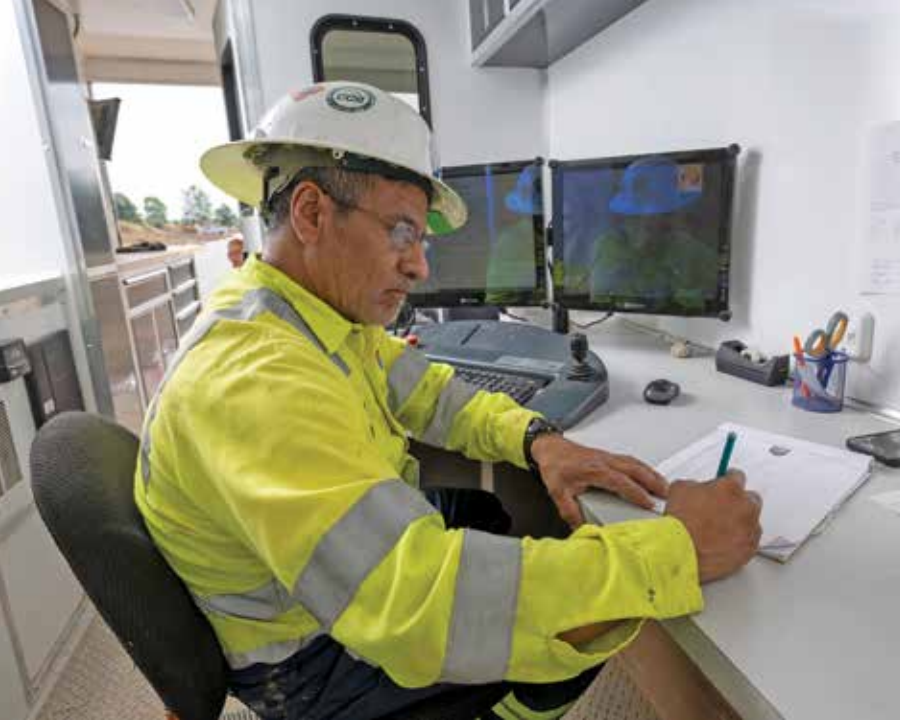
« Freddy Garcia operates a RapidView IBAK mainline system during a post-cleaning inspection in Greenfield, Indiana.
