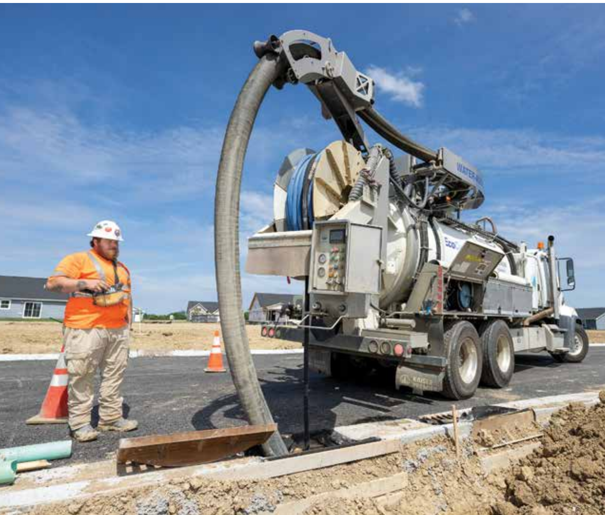
« Heavy-equipment operator David Beeman Fonseca uses a Kaiser Premier EcoCycler on a job in Greenfield, Indiana.
