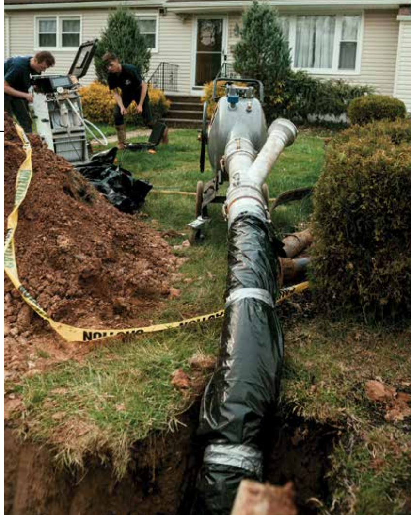
▲ Luis Fanlo says his company can do two pipe lining jobs per day thanks to the Sewertronics SpeedyLight+ lining system’s LED light technology, which can cure liners at a rate of up to 3.3 feet per minute.
