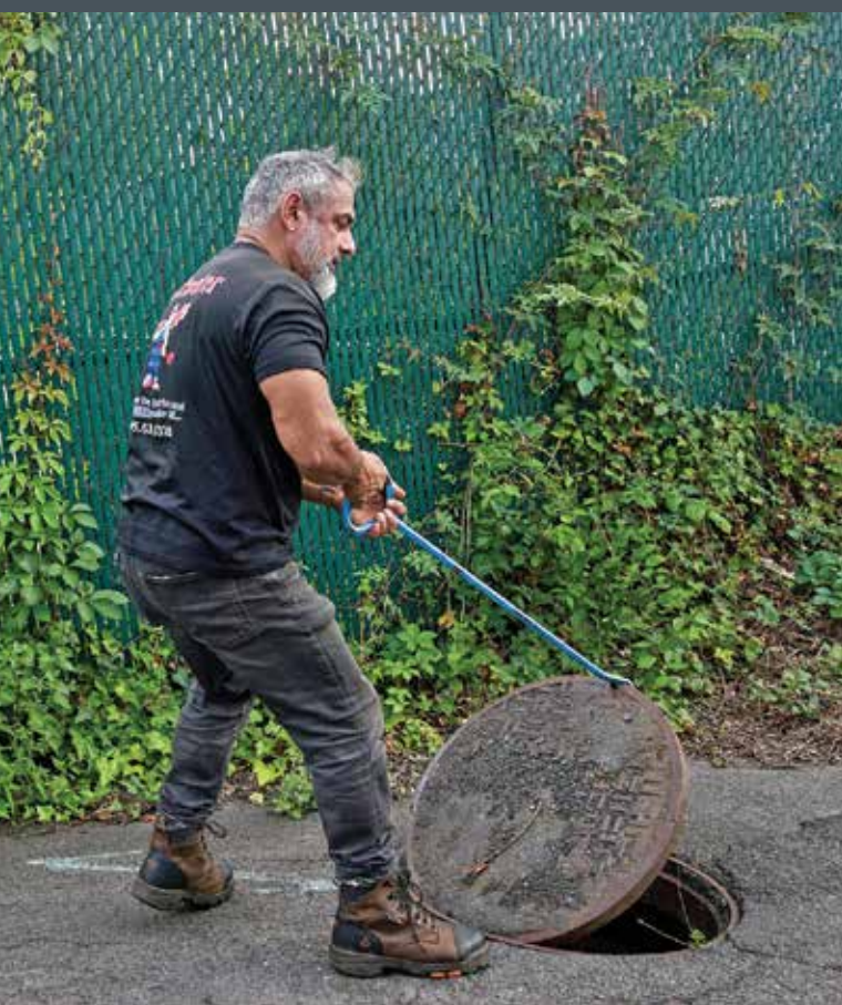
▲ Tony Garcia is one of two full-time technicians working for Dr. Rooter and owner Dave Ferrier. He uses a T&T Tools hook to access a manhole.
