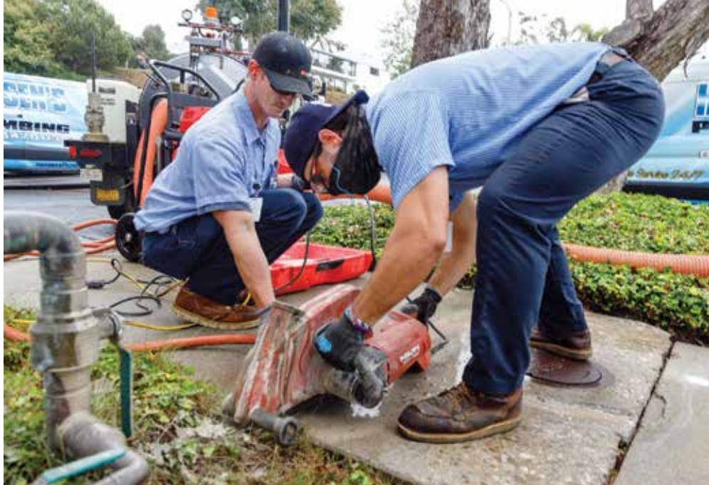
▲ Avery Brooke and Josiah Cagan use a Hilti DCH 300-X electric cutter to cut through sidewalk during a sewer line repair.
