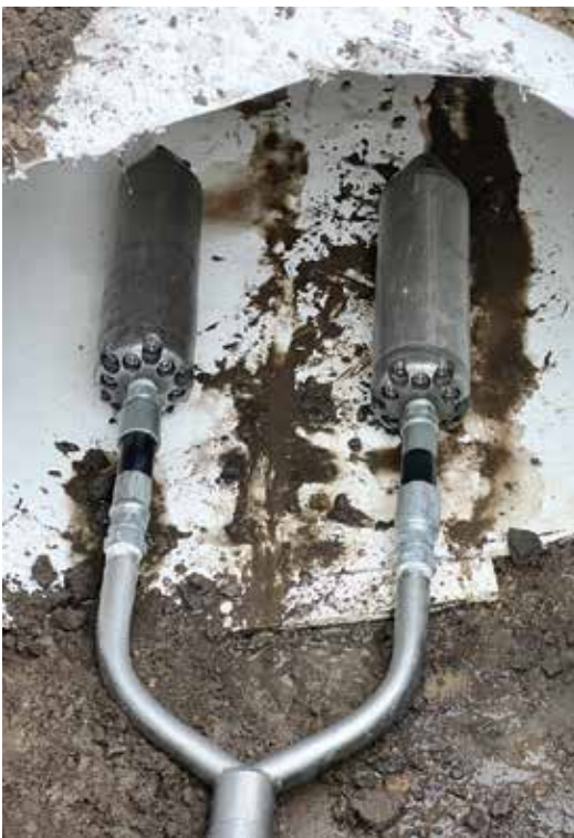
⚡ A twin jetter setup using OMG nozzle heads from KEG Technologies helped crews handle challenges with cleaning the box culverts.
