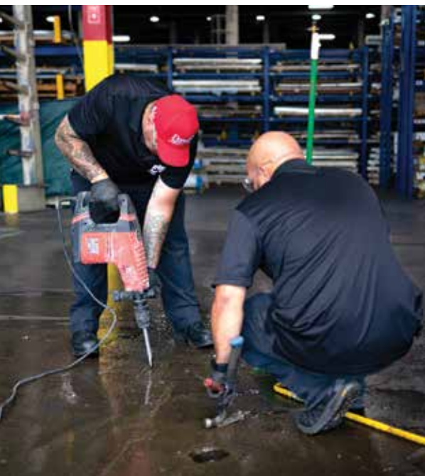
▲ Daniel Gallagher uses a chipping gun to remove a drain cover while Juan Roman looks on.
