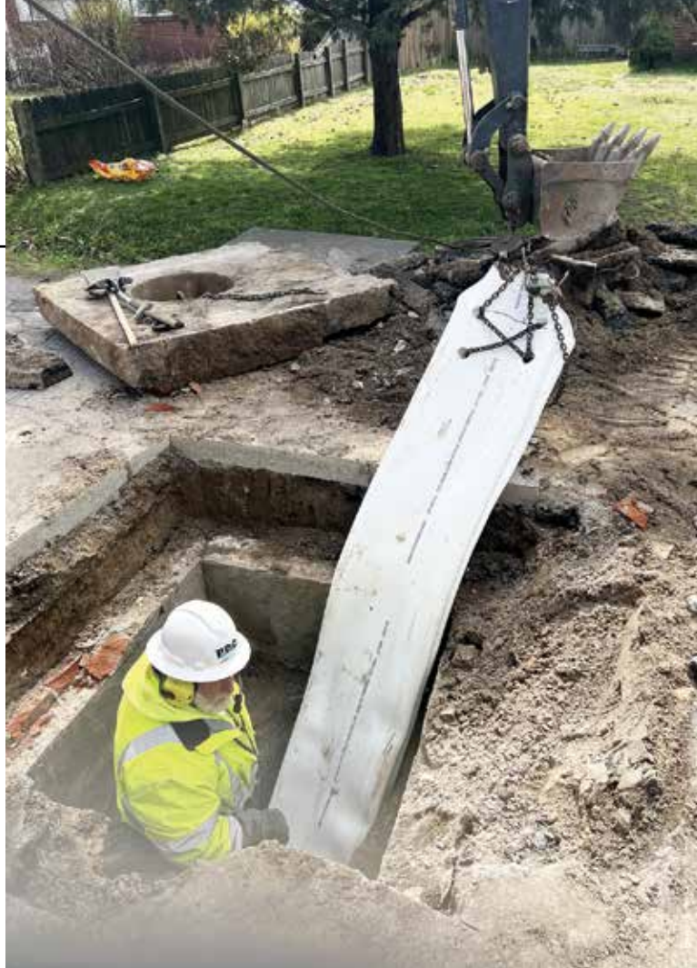
▲ Pipeline and Drainage Consultants out of Kentucky took on the job, lining 1,140 feet of the 10,000 feet of old box culverts that run throughout Kennett.
