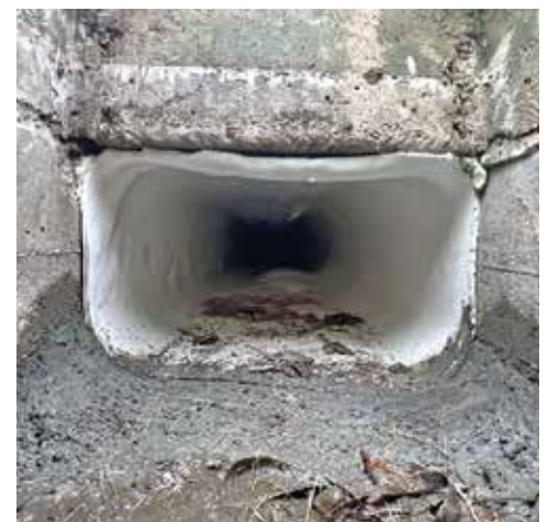
⚡ A culvert after being rehabbed with Warrior Trenchless Solution's Thermoform liner product.
