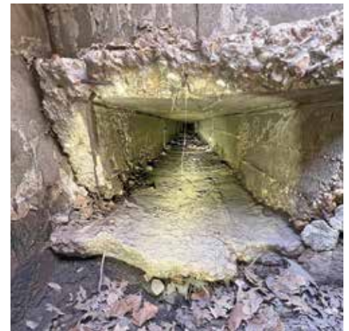
⚡ Kennett, Missouri, officials worried that deteriorating 1930s era box culverts could cause problems.
