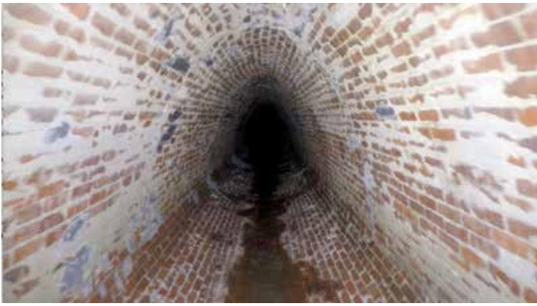
◀ Before: The view of an egg-shaped culvert in Lakewood, Ohio, before it was rehabbed by Marra Services with the Quadex I-MARS spray-lining system.
