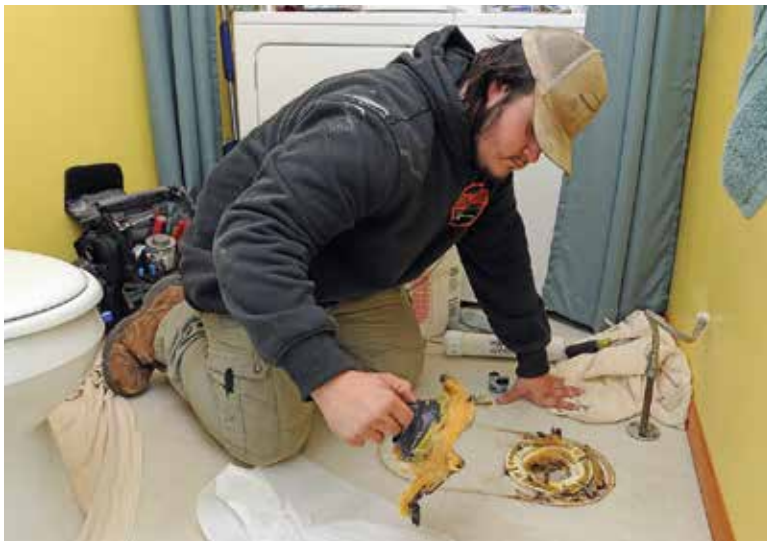
« Apprentice Zach Bajewski cleans the old wax ring off before a new wax ring and toilet are installed in a home in Cudahy, Wisconsin.
