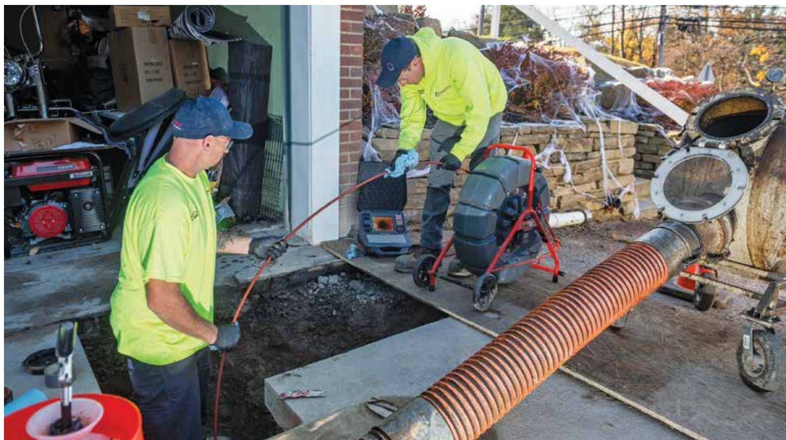
✓ Mike DiSanto and Dylan Belfiore of Matt Mertz Plumbing complete a trenchless sewer repair in Pittsburgh.
