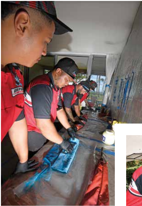
◀ Allens Plumbing crew members prepare to coat a sewer line on the island of Maui.
