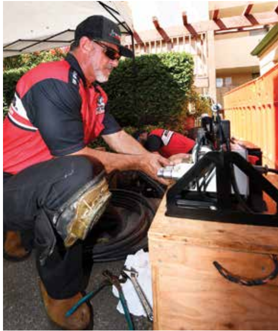
▶ Allens Plumbing division manager Ken Davis sets up a hydraulic ram while preparing to pull a bursting head and new section of pipe through a sewer line at a condominium on the island of Maui.
