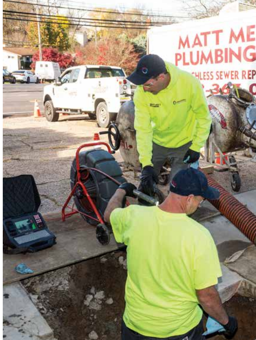
▲ Belfiore and DiSanto use a RIDGID SeeSnake pipeline inspection camera on a trenchless sewer repair job as Matt Mertz looks on.
