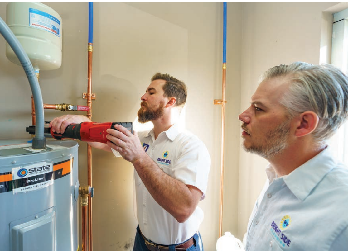
➤ Barker uses a Milwaukee M18 press tool on a water heater installation job.
