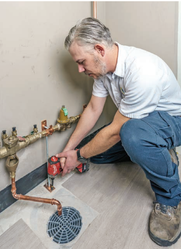
▲ Bright Side Plumbing apprentice James Gardner uses a Milwaukee Tool driver to secure a cover at a water heater installation job.
