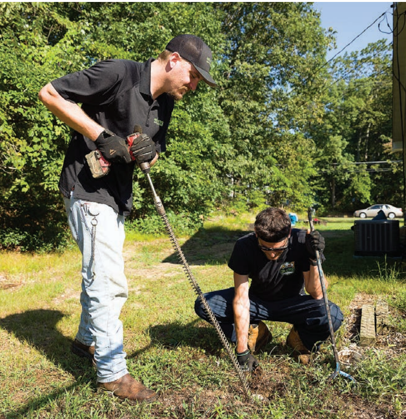
Steve Russo and Kraemer use a Milwaukee drill to snake out a septic system at a home in New Egypt, New Jersey.
