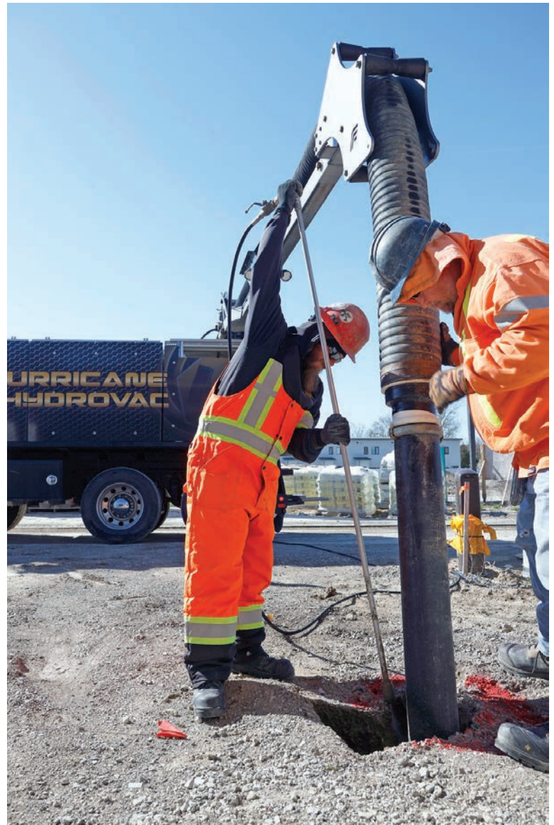
Operators Carmon Geffs and Tom Ross use a Foremost hydrovac to locate a utility line on a job site in Windsor, Ontario.
