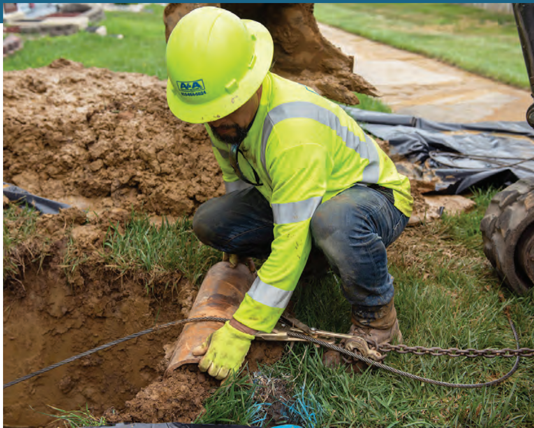
➤ Raul sets up pipe bursting equipment to replace a residential water service line.
