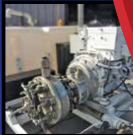
Preventative Maintenance & Pump Rebuilds
