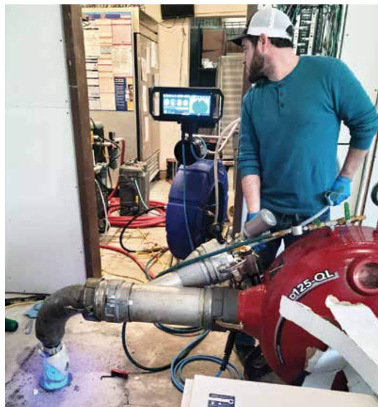
Underground Pipe Co. lining technician Richard Schneider monitors the HammerHead Trenchless Bluelight LED system as it cures a sewer liner.
