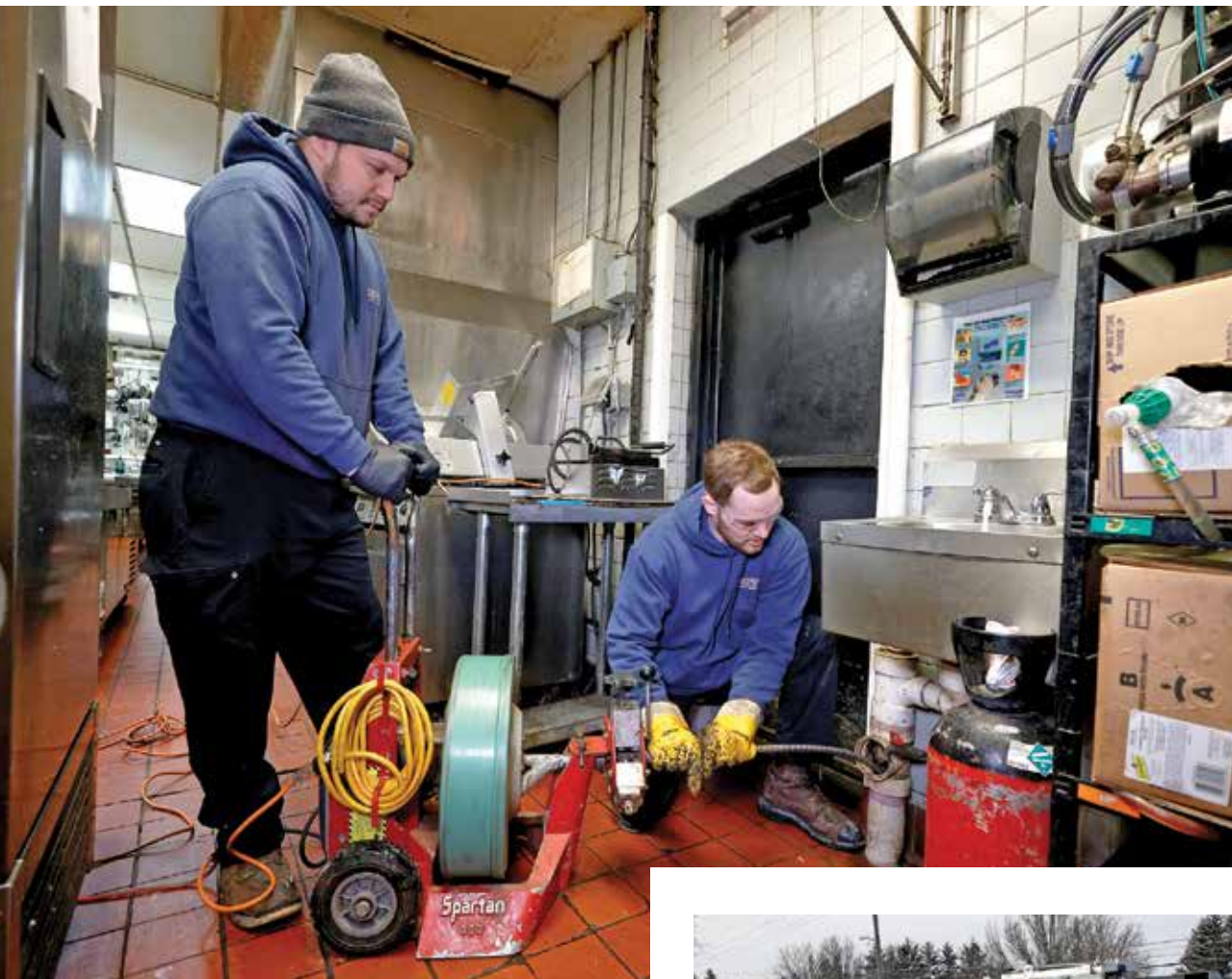
« Service Pro technician Sean O’Keefe uses a Spartan Tool drain machine to clear a drainline at a restaurant in Northville, Michigan.
