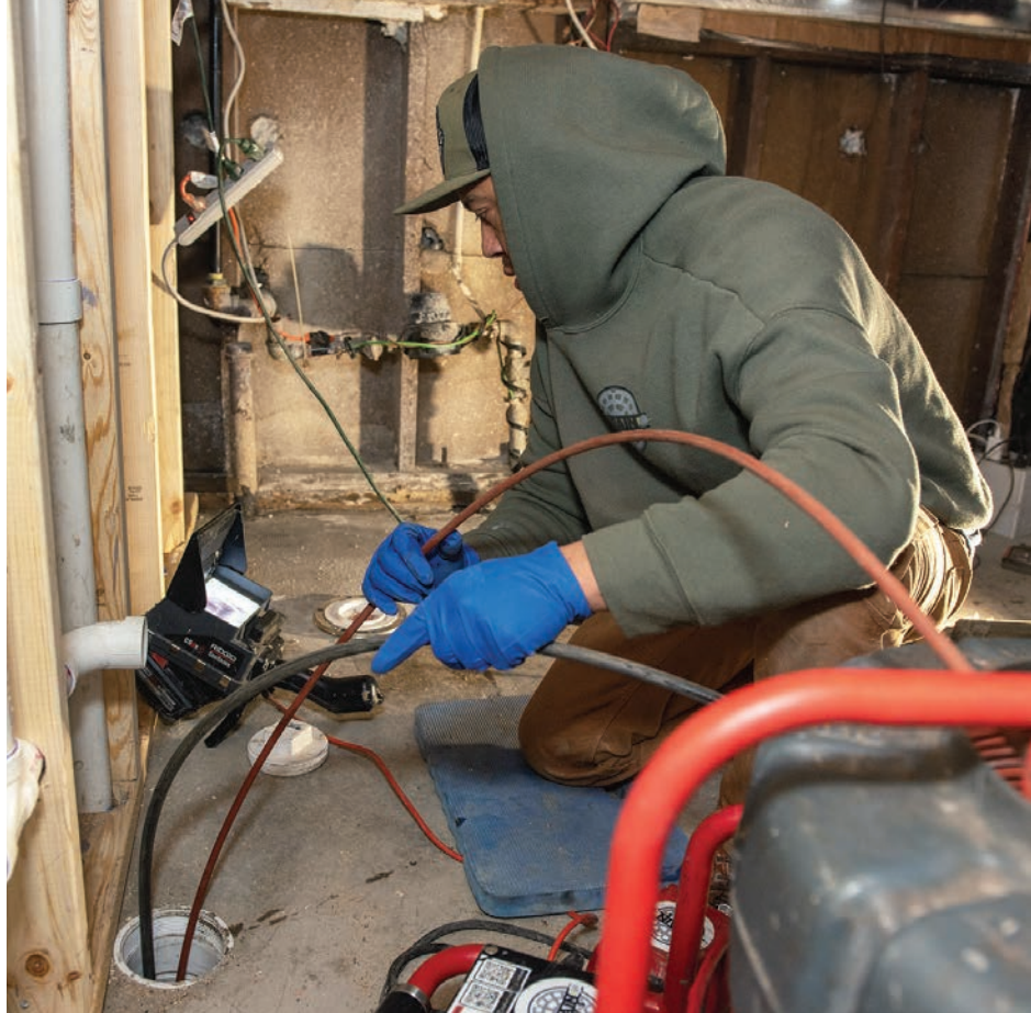
Delgadillo's Chicago-based company does descaling work nearly every day due to the city's older, cast iron pipes.
