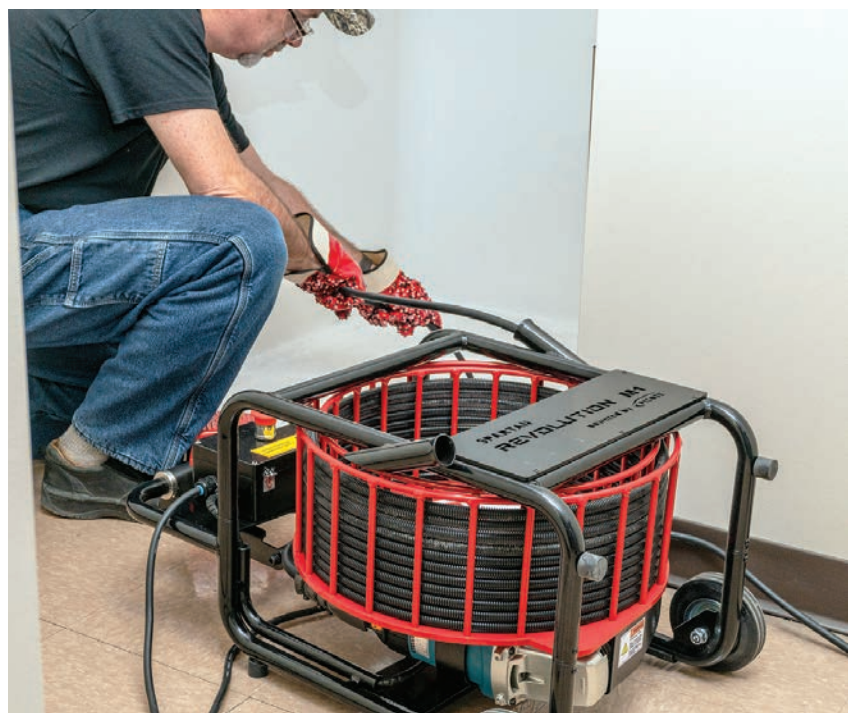
Flexshaft machines are designed for fast and efficient drain cleaning, including the removal of soft blockages, scale, calcium buildup, tree roots and concrete. Here a contractor uses a Spartan Tool Revolution M1 to clear a drainline.
