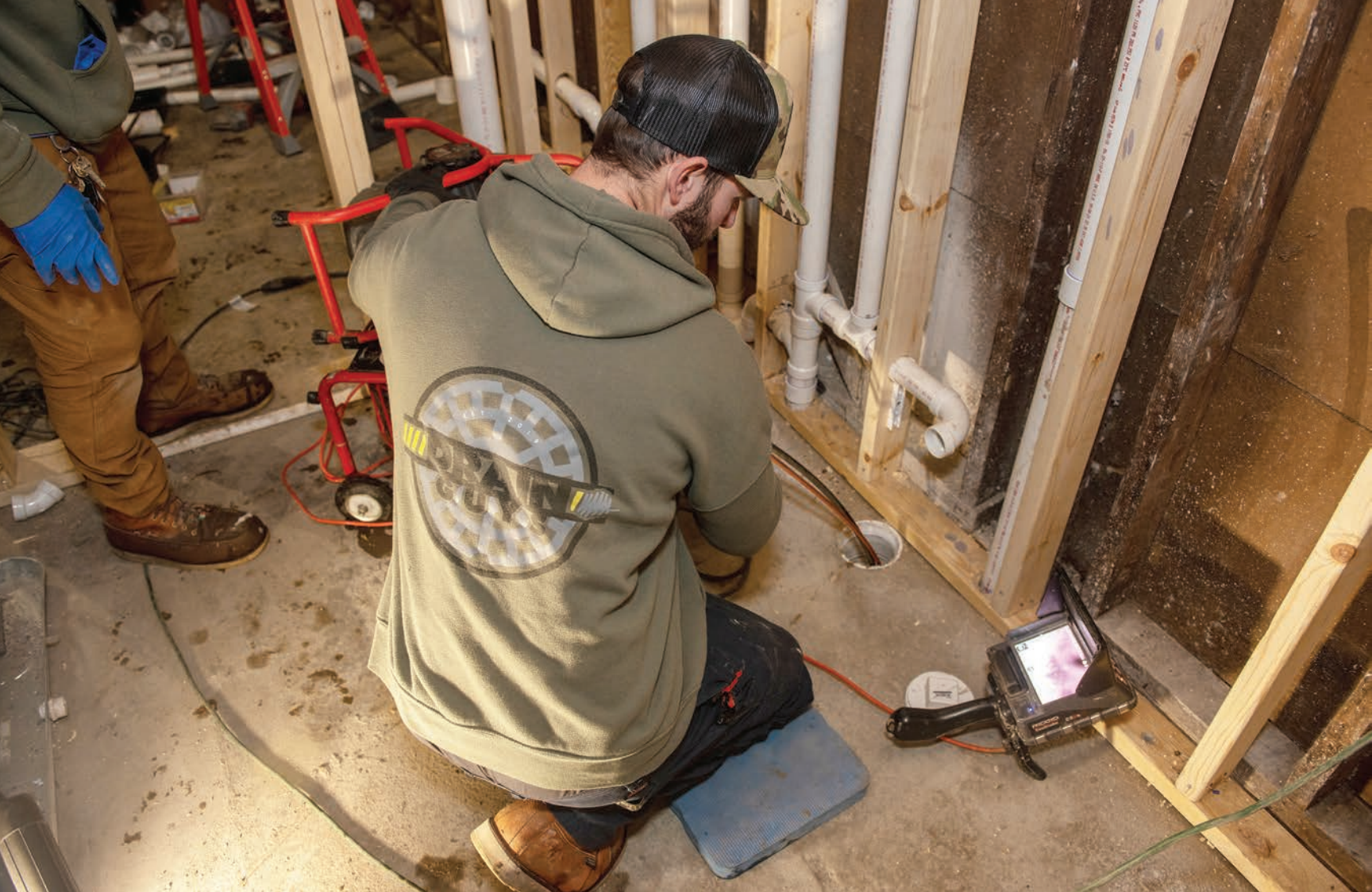
🔧 Technician Bill Oudshoorn uses a Picote Mini Miller to descale a drainline, while watching the progress with a RIDGID SeeSnake.
