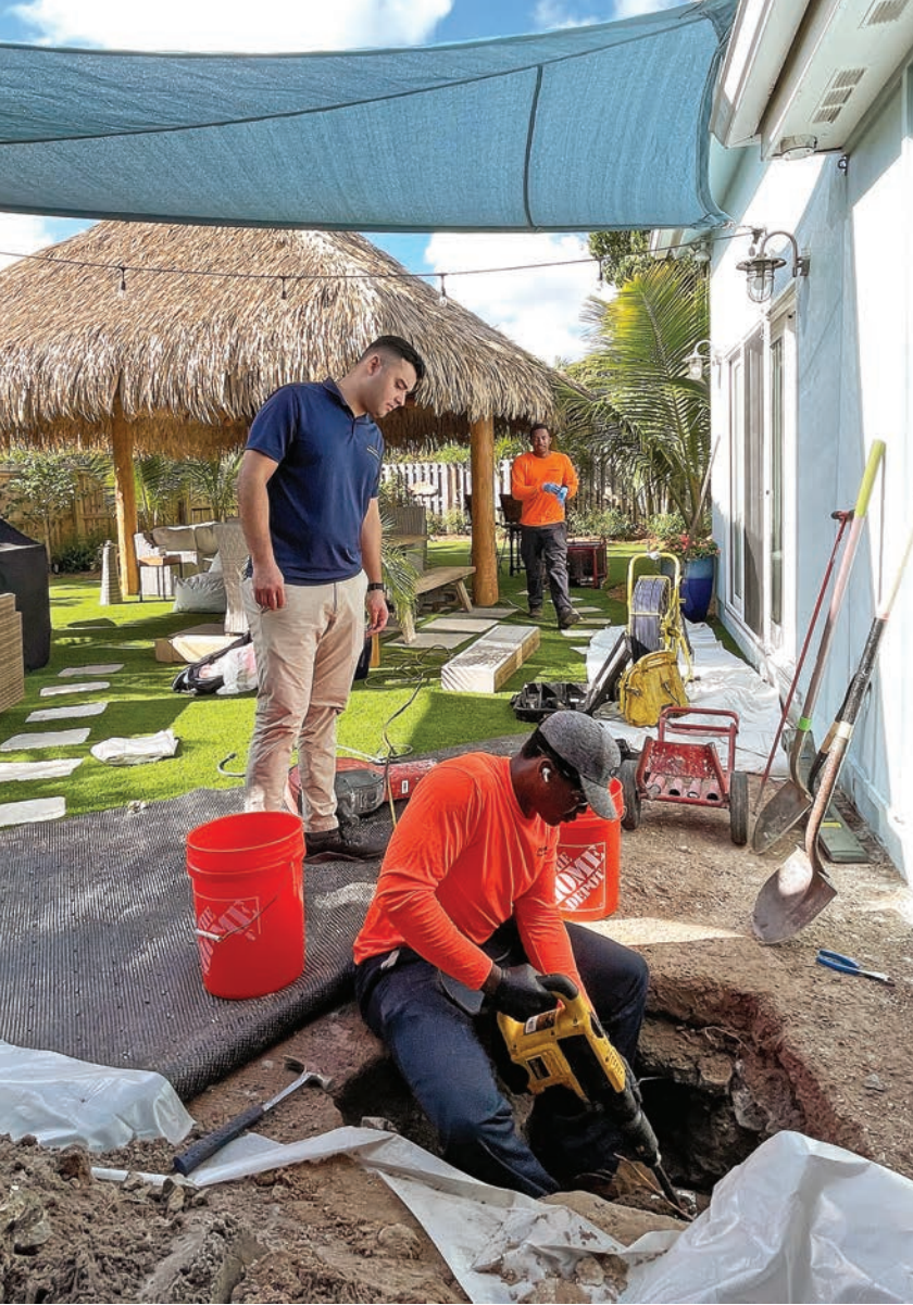
📍 Jones breaks up rock to expose a pipeline in the access pit.
