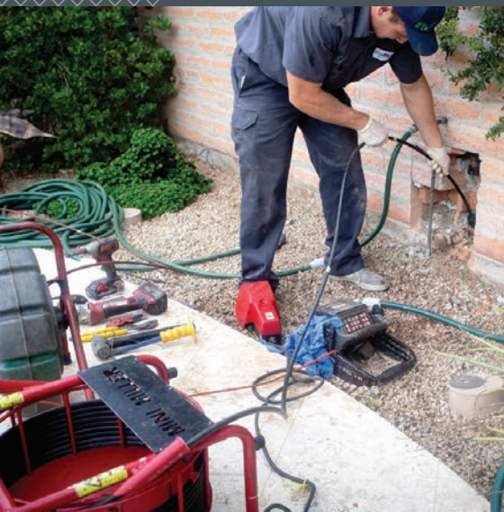
▲ NuFlow Services technician Kolten Tescher uses a Picote Mini Miller to clean out a drainline on a job in Paradise Vally, Arizona.
