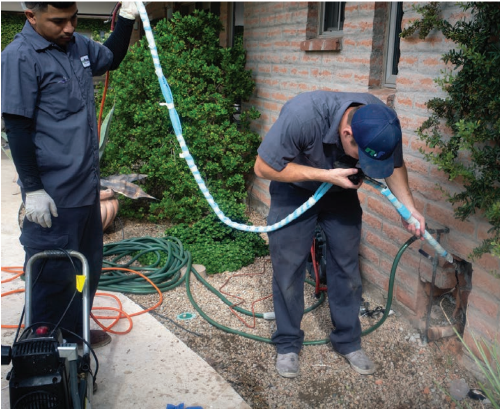
Technicians Rivera (left) and Tescher install a NuFlow liner through a clean-out.
