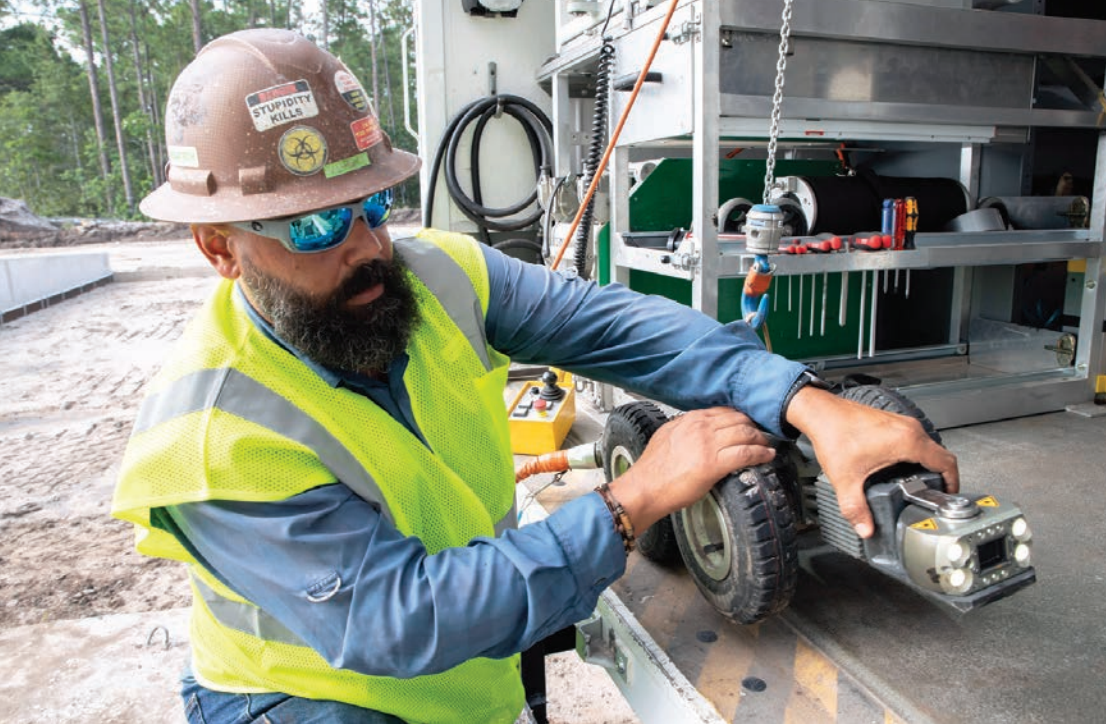
« Technician Manny Rivera prepares a Rausch KS135 robotic camera to do a video inspection of the new storm drains at a warehouse in Orlando.
