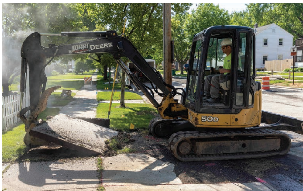
👉 Mark Joski lifts out a section of sidewalk for a residential sewer job in Green Bay, Wisconsin.
