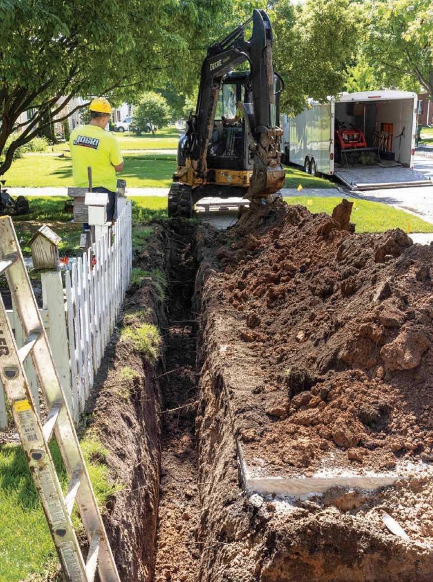
« The Joski Sewer Services team prepares a trench for a new residential sewer connection in Green Bay.
