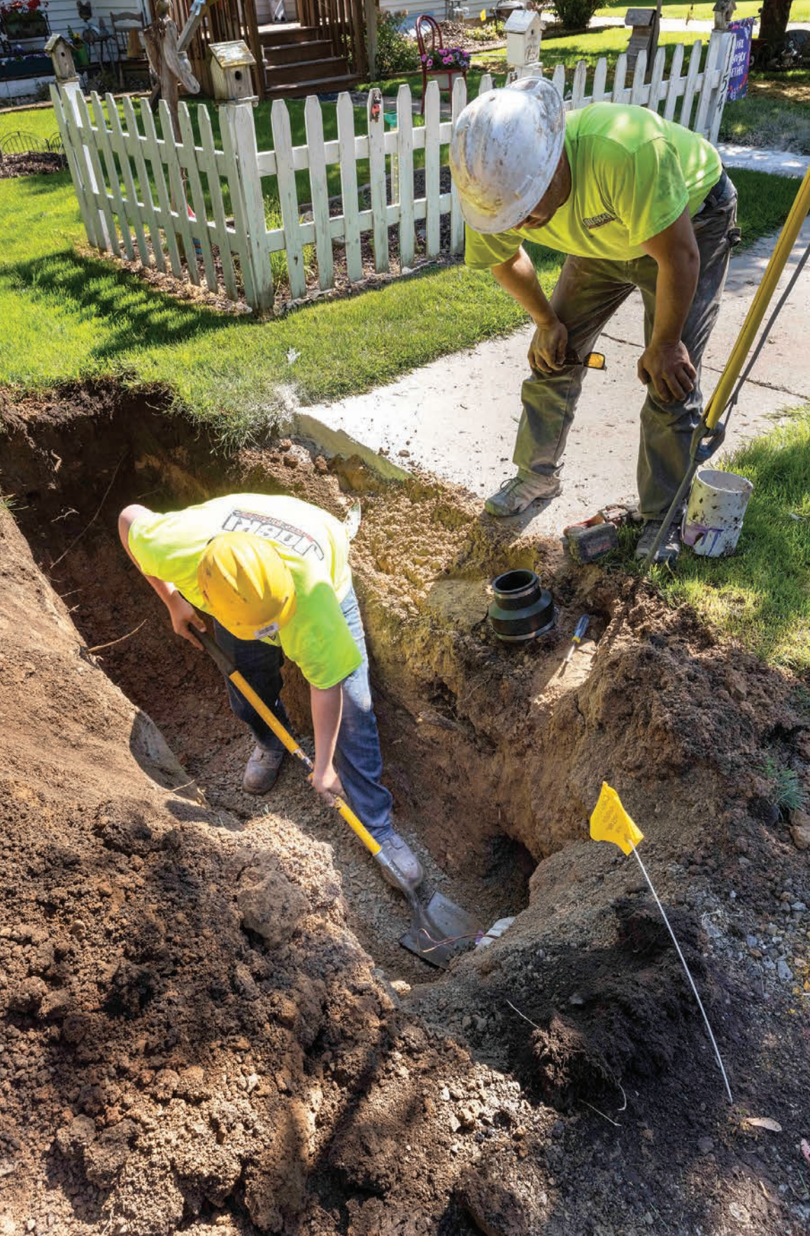
◀ Masen Block prepares a residential storm sewer connection while Joski looks over his work
