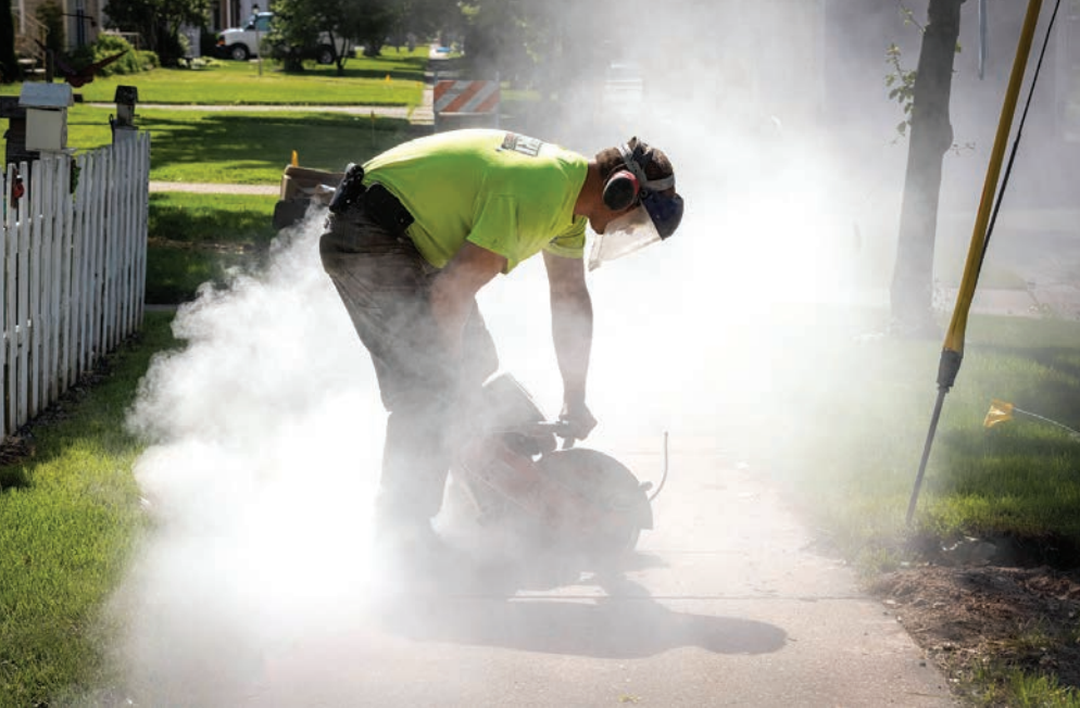
◀◀ Joski cuts out a section of a sidewalk with a Husqvarna K760 Cut-n-Break concrete saw.
