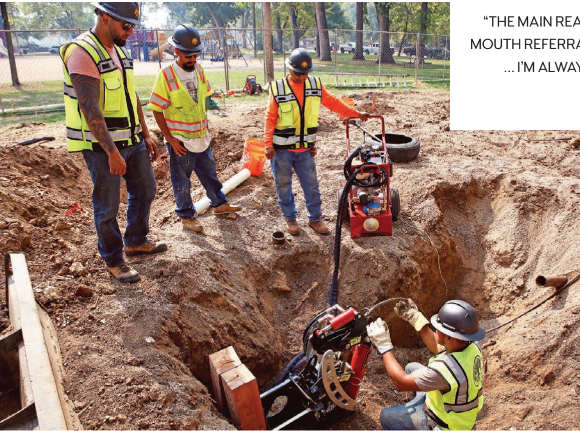
Technicians (from left) Anthony Ibarra, Luis Castelar Trulljo and Kirino Pacheco Luna watch as Jose Pacheco Luna makes an adjustment to the pipe bursting machine in the pit.
