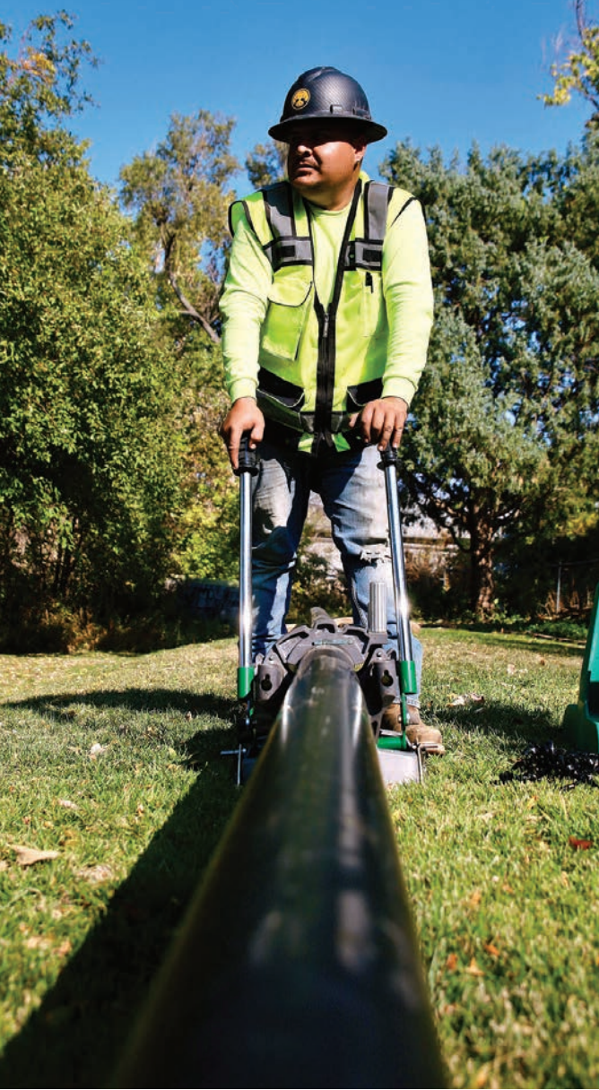
David Mendez uses a Pit Bull pipe-fusion machine to fuse sections of HDPE.
