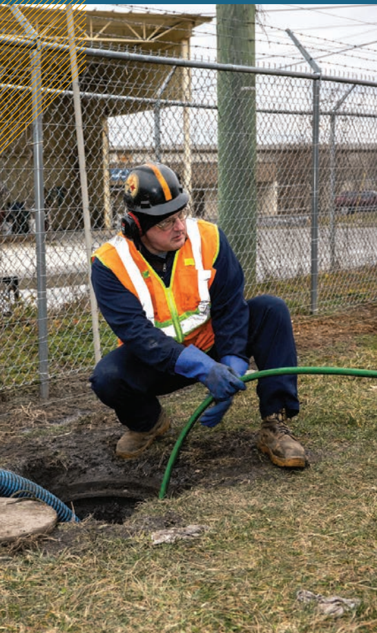
« Northstar Environmental Group VP of Projects James Kutzer helps his crew clean a storm drain.
