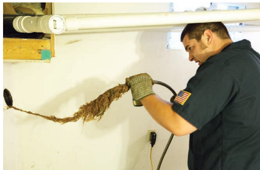
▲ A technician removes tree roots from a drain cable after clearing a sewer line at a residence. Root intrusions can be removed with either traditional drain equipment or a jetter, but using both makes the process much easier.
