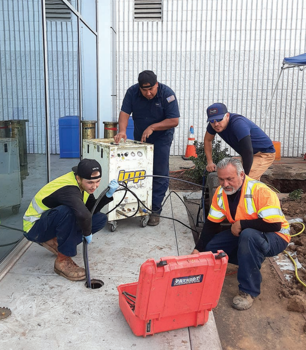
« Technicians Steven Parker, Pablo Miro, Pete Beccera and Santiago Tevino (from left) of Select Trenchless Pipelines watch the progress of the PipeCaster Pro pipe coating system from IPP Solutions.
