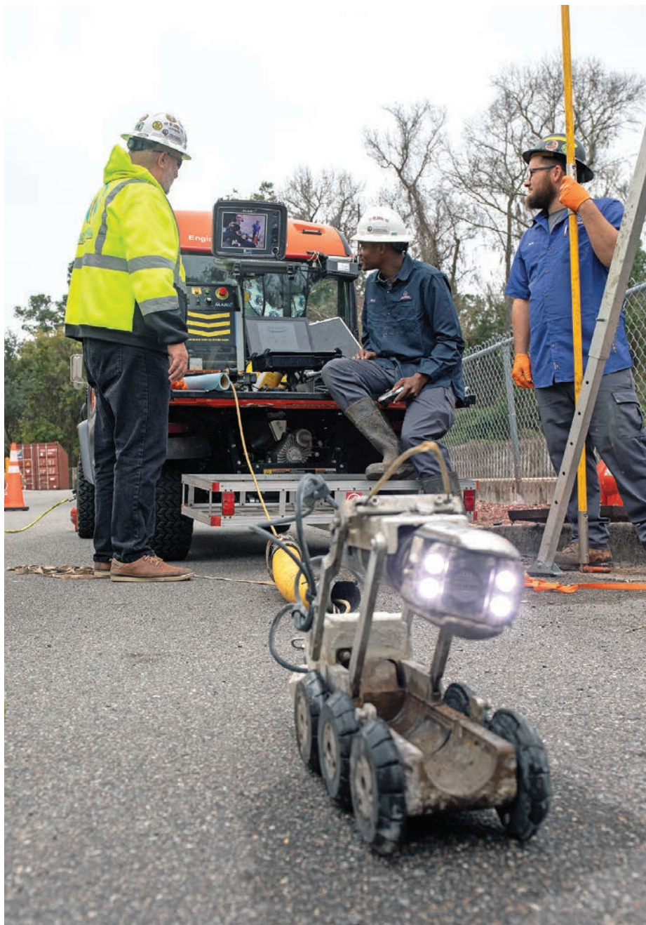
▲ Don Arch, Bernard Stafford and Buddy Blake (from left) check the video feed from a CUES Digital Universal Camera system before beginning an inspection.
