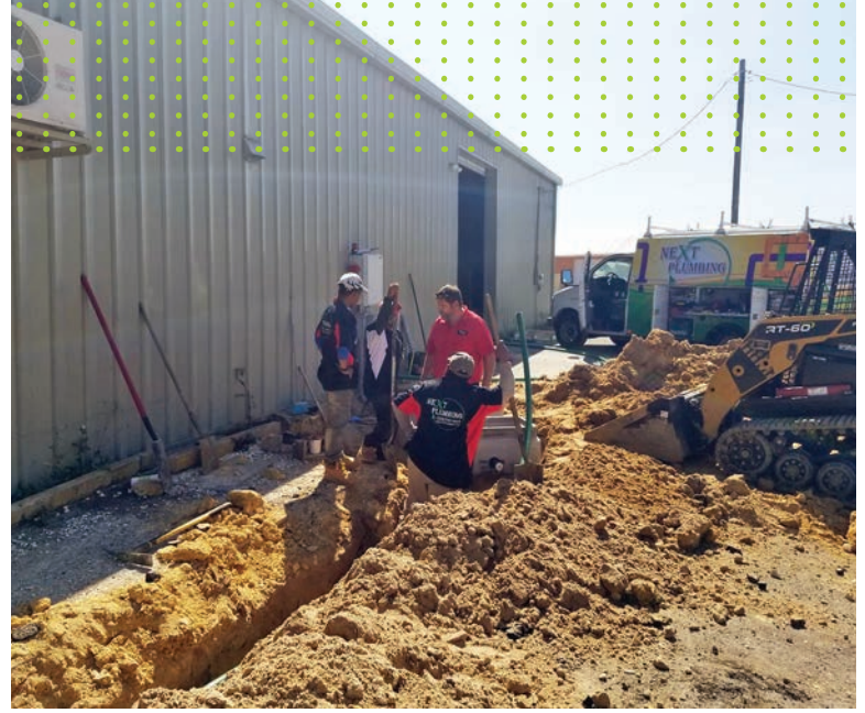
Next Plumbing crew members dig a trench to replace a wastewater line outside a commercial building.
