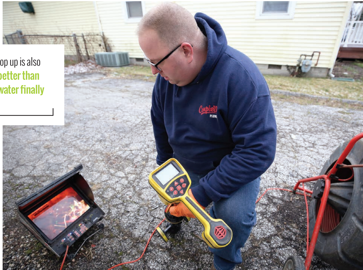
Haymer references the camera monitor while using a RIDGID SeekTech SR-20 locator to trace the path of a lateral line.
