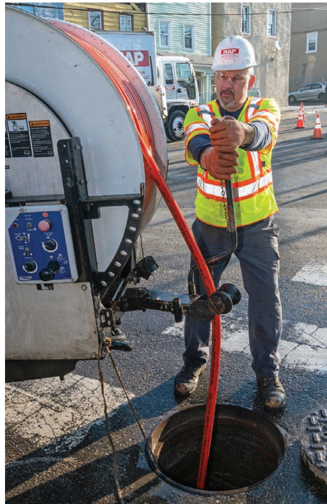
➤ Pleskowicz lowers the jetter hose into a manhole to clean the sewer line.
