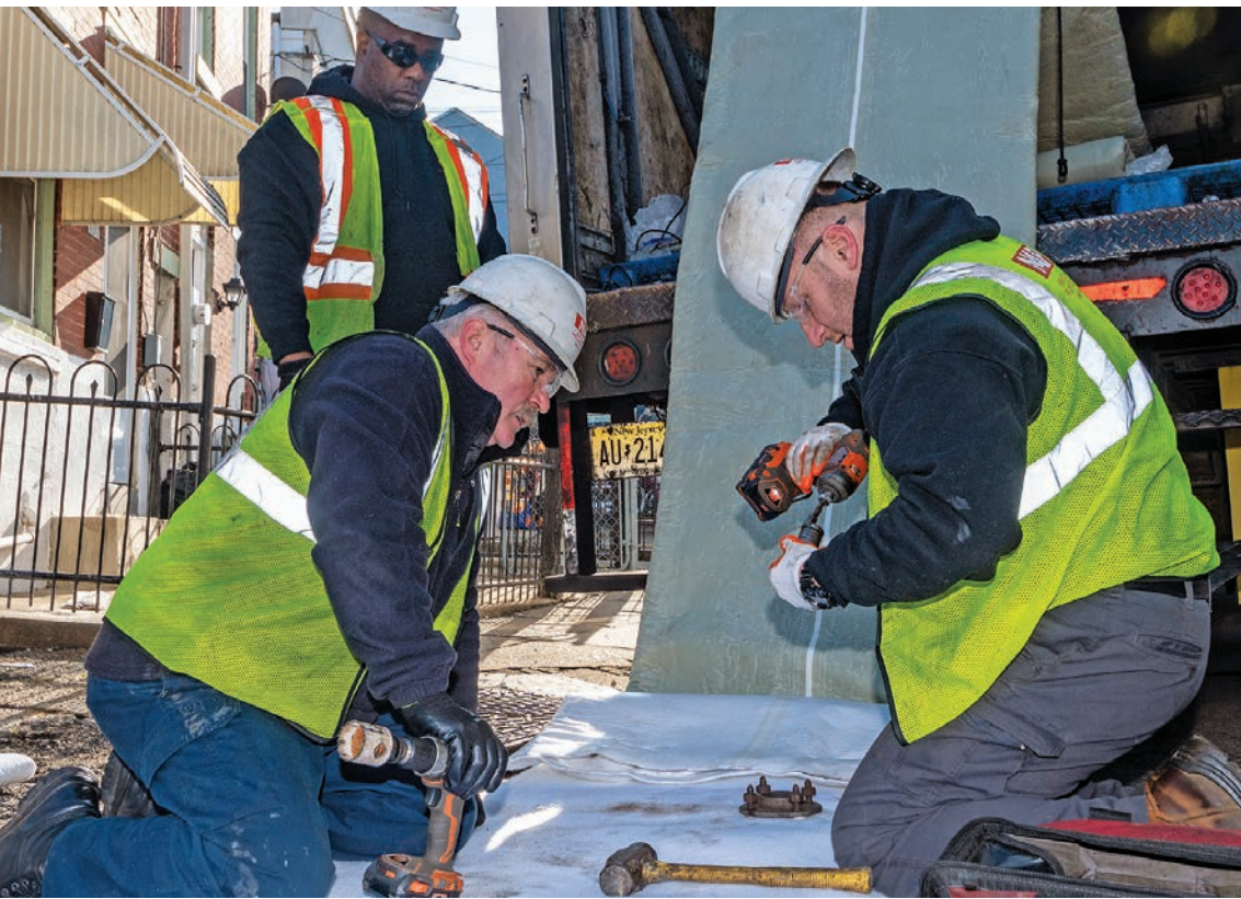
« Technicians James Bey (standing), Sławomir Kadlubowski (left), and Rafal Sasak prepare the Applied Felts liner for insertion into the manhole.
