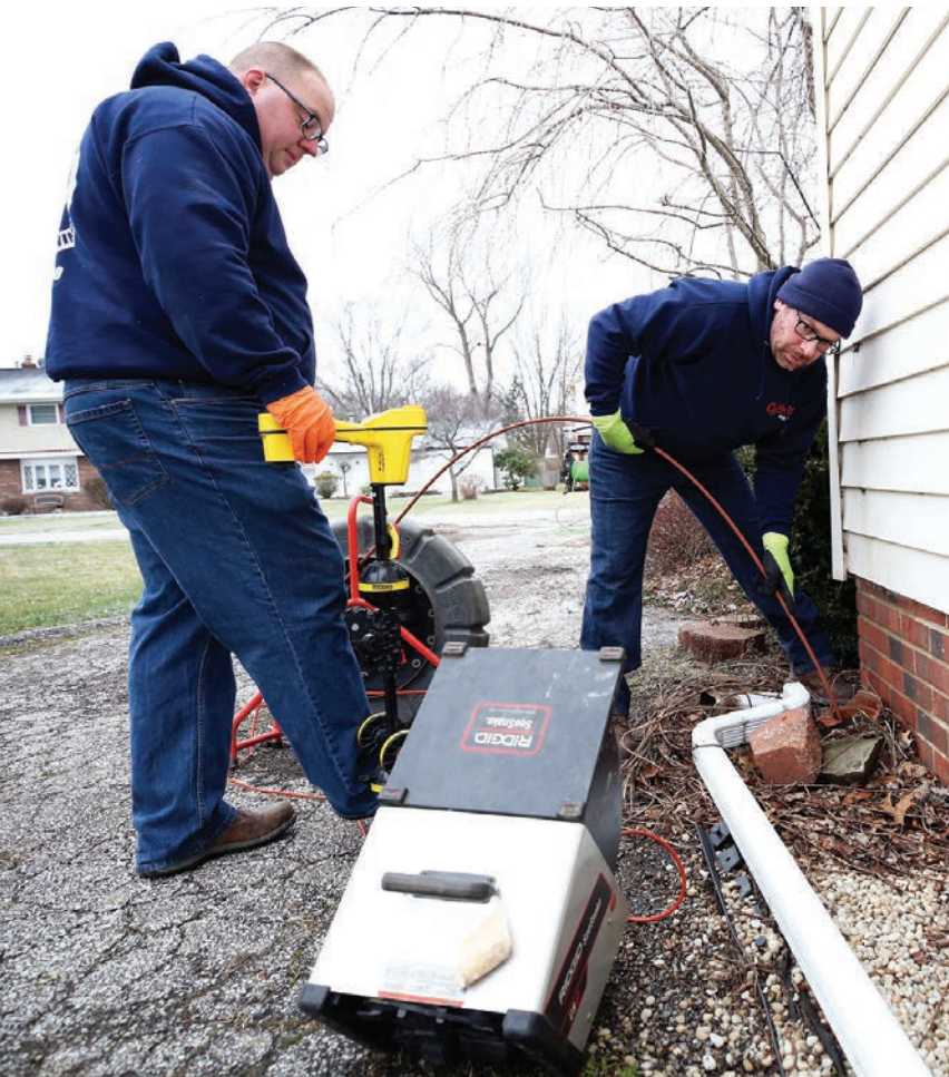
▲ Providing inspections helps show homeowners the condition of their lines along with any problems that may be present, which is helpful when discussing repair or rehabilitation options.
