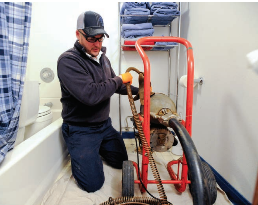
Joe Lienhard uses a RIDGID K-1500 sectional machine to clear a stoppage in a bathroom drainline.
