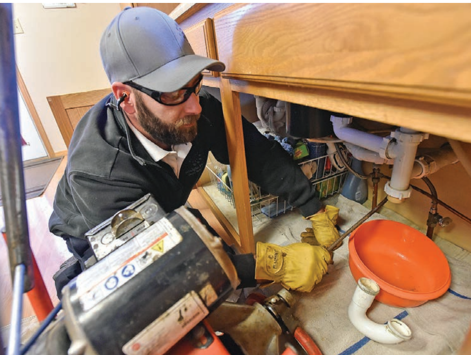
◀◀ Bradley Schwartz feeds cable from a RIDGID K-400 drum machine into a blocked sink drain.
