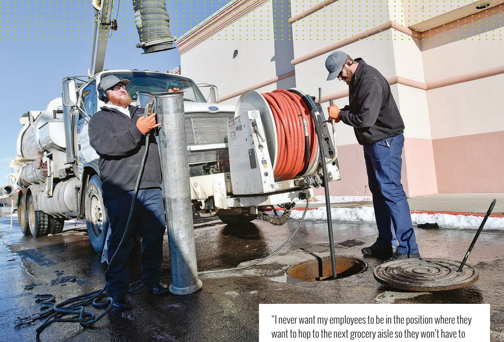
Technician Dennis O'Connell connects an extension tube to the Vector's vacuum boom while Zach Gloege cleans debris from a manhole.
