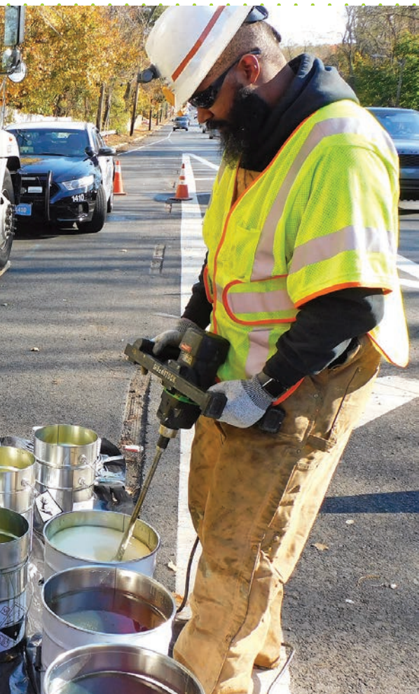
➤ Miguel Robles (left) and Kacy Wright mix buckets of two-part resin in preparation for lining a 42-inch cast iron host pipe.
