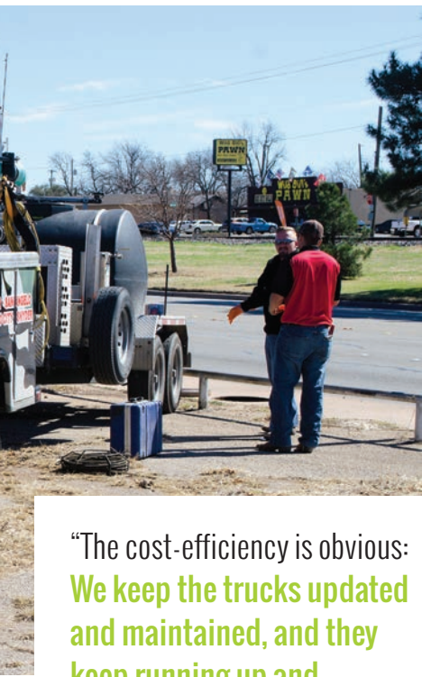
◀ A crew from Black Plumbing in Abilene, Texas, works on a job site in town. The company outfits each vehicle with GPS devices to track fuel usage and time on jobs in an effort to boost efficiency. (Photography by Cory Jones)
