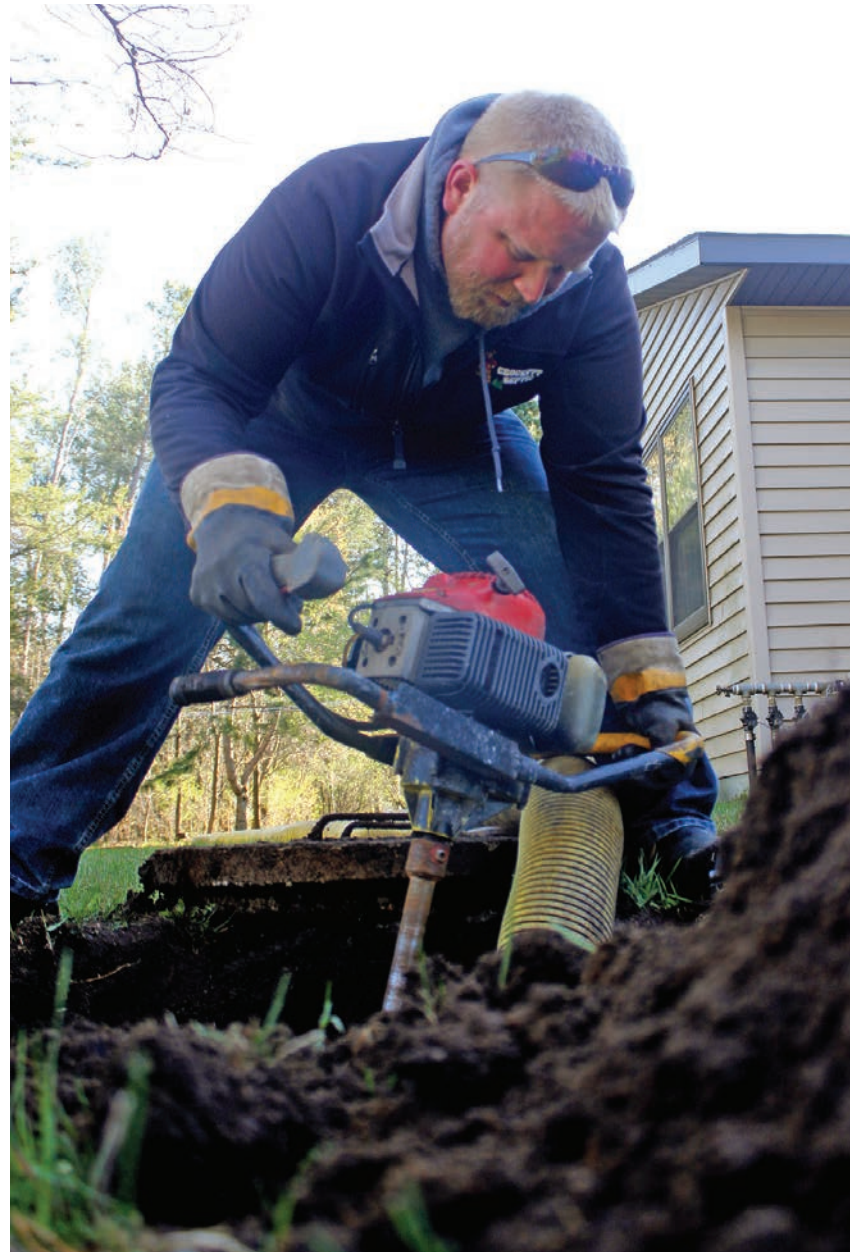
Using a Crust Buster to break up the solid material in the septic tank before pumping it out helps make sure the tank is properly emptied.
