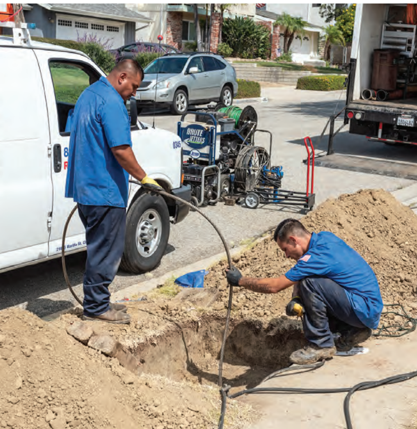
📍 Miro (left) and Vella monitor progress in the receiving pit as new pipe is pulled into place.
