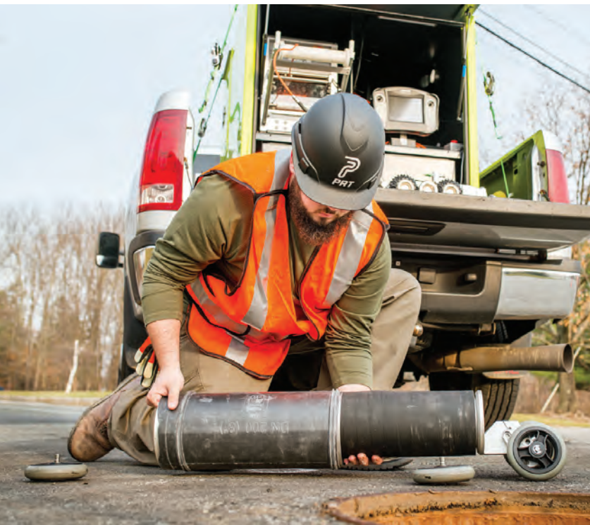
▲ A technician slides the Quick-Lock sleeve and rubber gasket onto the four-wheeled packer, which is then pushed into position by a robotic camera. (Photos courtesy of Pipeline Renewal Technologies)
