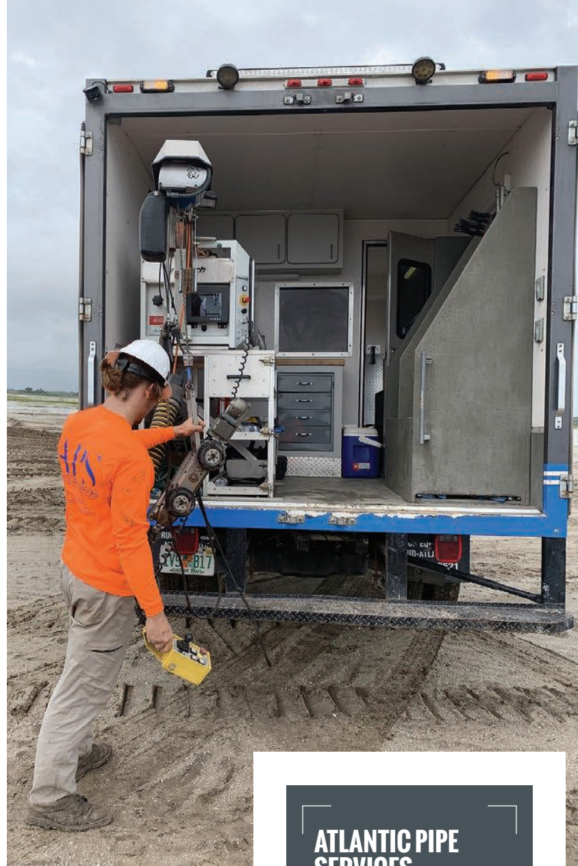
▲ Atlantic Pipe Services technician Chad Comis uses a winch to load the Rausch M-Series KS 135 laser profiler into a camera truck on a road-construction job site in Florida.
