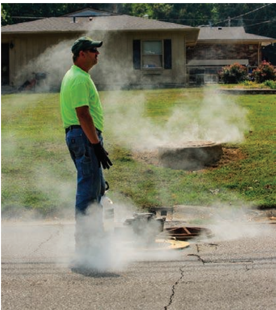
◀◀ A utility crew member operates a Hurco Technologies smoke-testing machine at a manhole, and then watches for smoke to appear.
