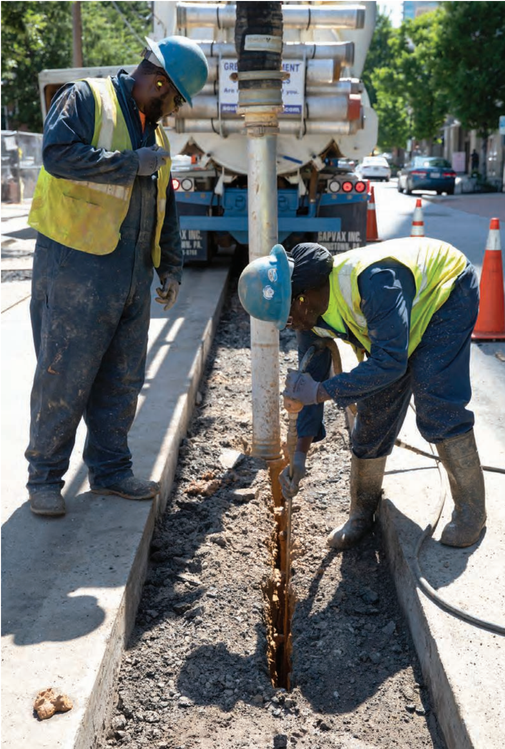
◀ Cedric Watson (left) and William Dubose use a GapVax hydroexcavator to locate buried utility lines.
