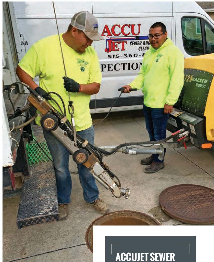
⤴ Cutter operator Lorenzo Tapia (left) and camera operator Pedro Funes get set up to clear out a line with the Schwalm Talpa FSR 2060 robotic cutter system.
