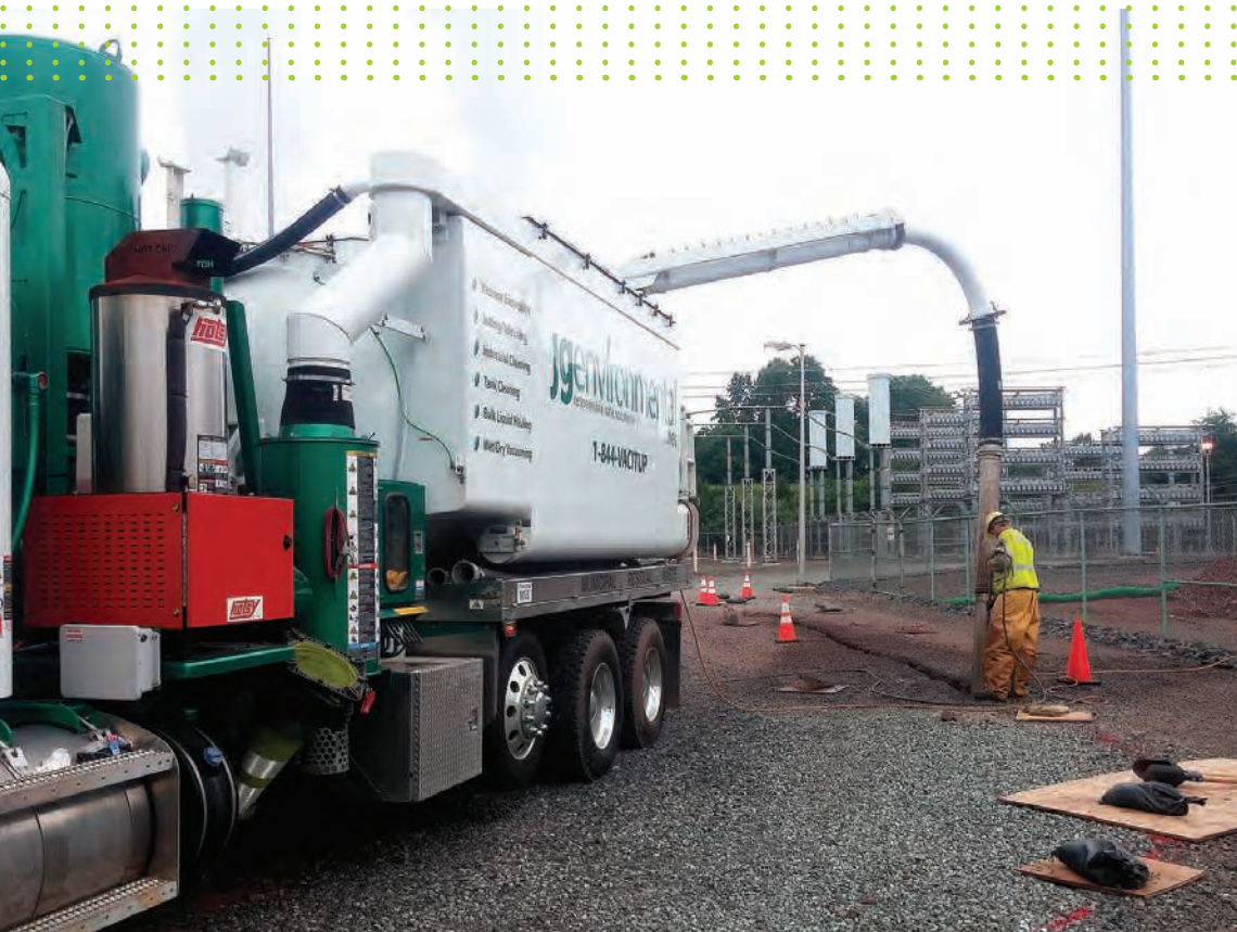
The new GapVax hydroexcavator is ready to work at a job site in Lancaster, Pennsylvania.
