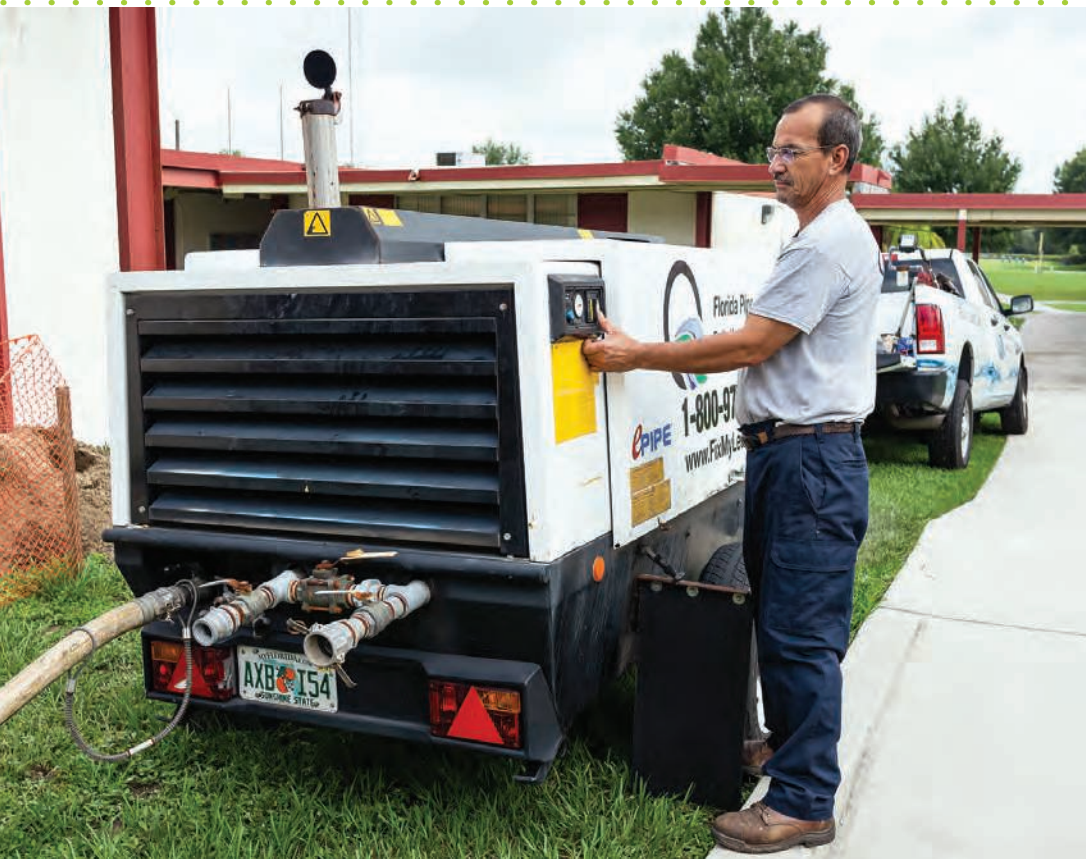
➤ Technician Javier Martinez checks an AtlasCopco compressor during an ePIPE restoration project.
