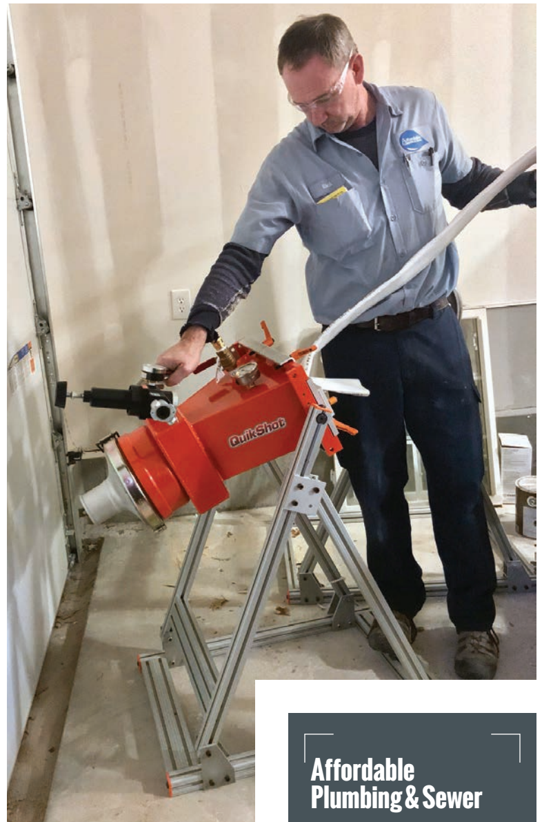
▲ Rick Ramsey, owner of Affordable Plumbing & Sewer in Kansas City, Missouri, feeds a liner into a Quik-Shot inversion unit on a lateral lining job.
