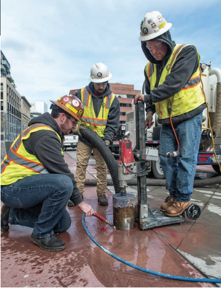
Josh Allen, Michael Griego and Scott Canadas (from left) drill a concrete core in a sidewalk in downtown Denver to reach a buried utility line.
