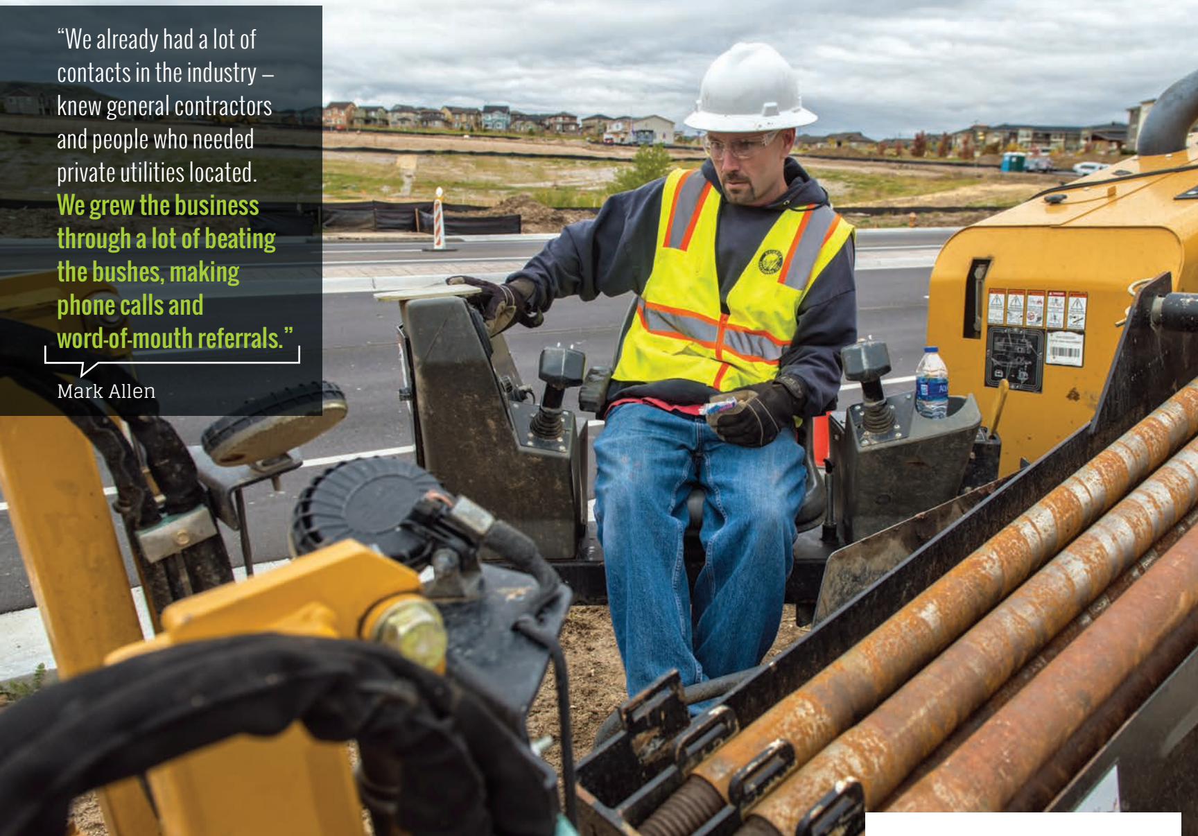
Branden Witt, head locator with Diversified Underground, lines up a Vermeer D20X22 horizontal directional drilling unit in preparation to install underground electrical utilities for new traffic lights.
