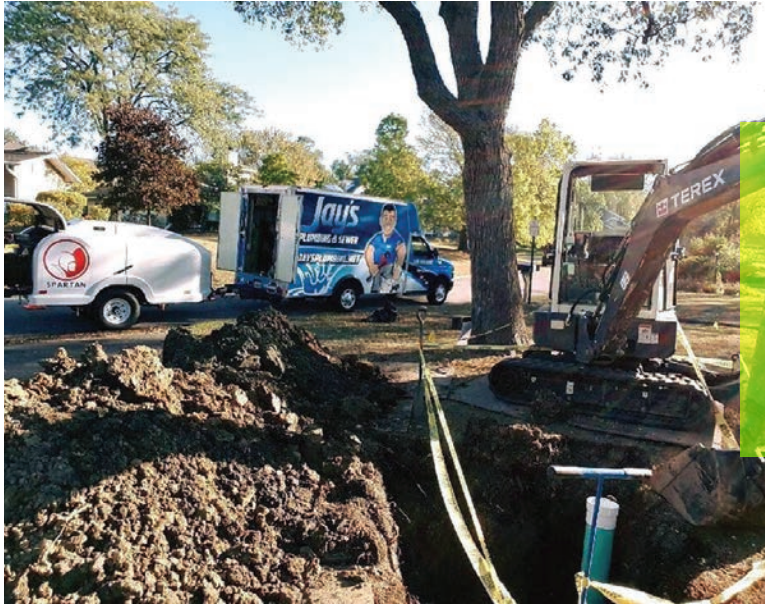
◀ A crew works on the installation of a new lateral line clean-out at a residence in Downers Grove after jetting the line with a Spartan trailer jetter.
