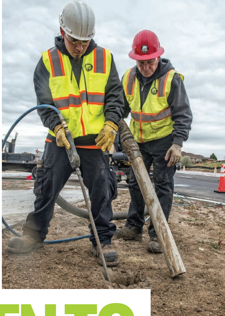
◀ Rudy Padilla (left) and Mike Canandy of Diversified Underground use a Vermeer vacuum excavator to expose an underground electric line.
