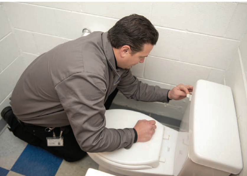
✦ Mike Krejci works on a toilet repair at a commercial job site in Downers Grove.
