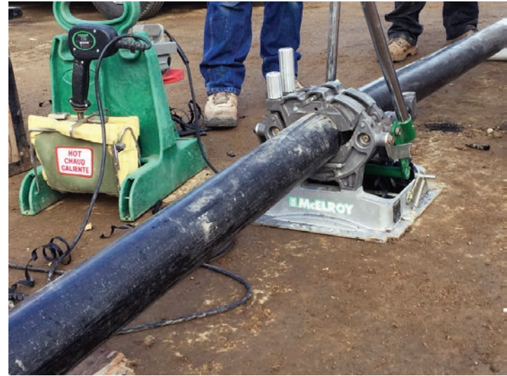
✔ Subcontractors use a McElroy fusion machine to join segments of HDPE pipe on a line replacement job.
