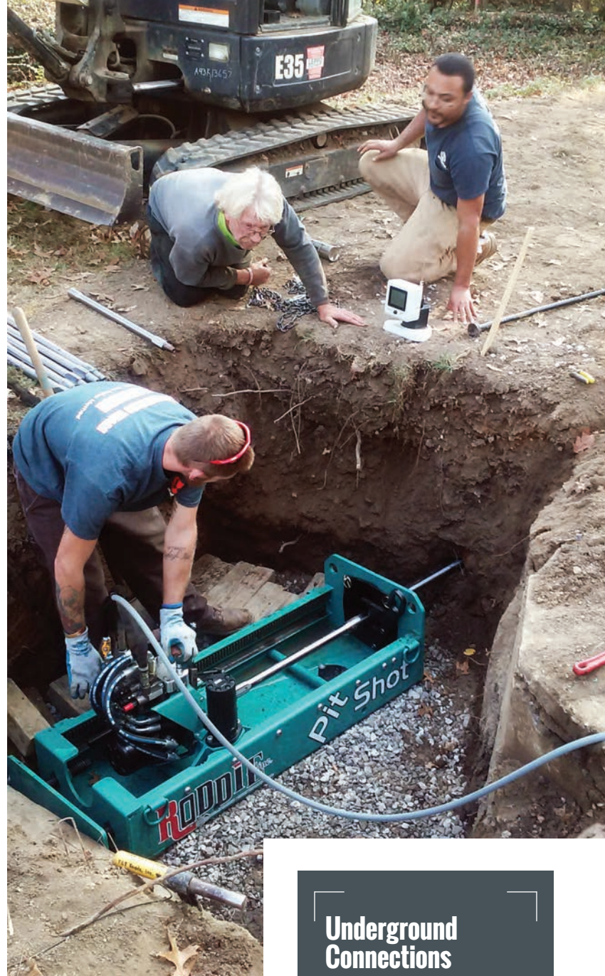
Andrew Jackson of Underground Connections runs the RODDIE Pit Shot directional drilling machine while foreman Clark Kinney (center) and Jeremiah Kinney help from outside the pit.
