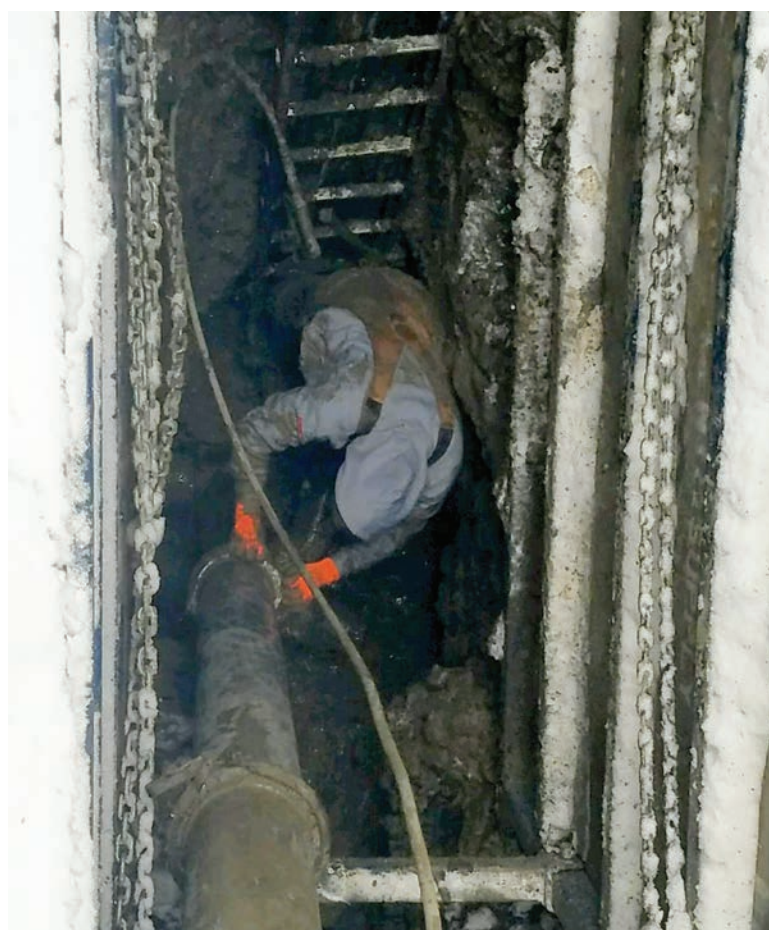
A worker hydroexcavates to expose a utility line in a shored trench.
