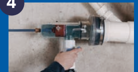
OPEN VALVE AND DRAIN CONTENTS
