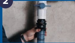
ATTACH DRAIN HOSE
