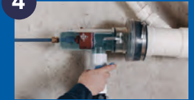
OPEN VALVE AND DRAIN CONTENTS
