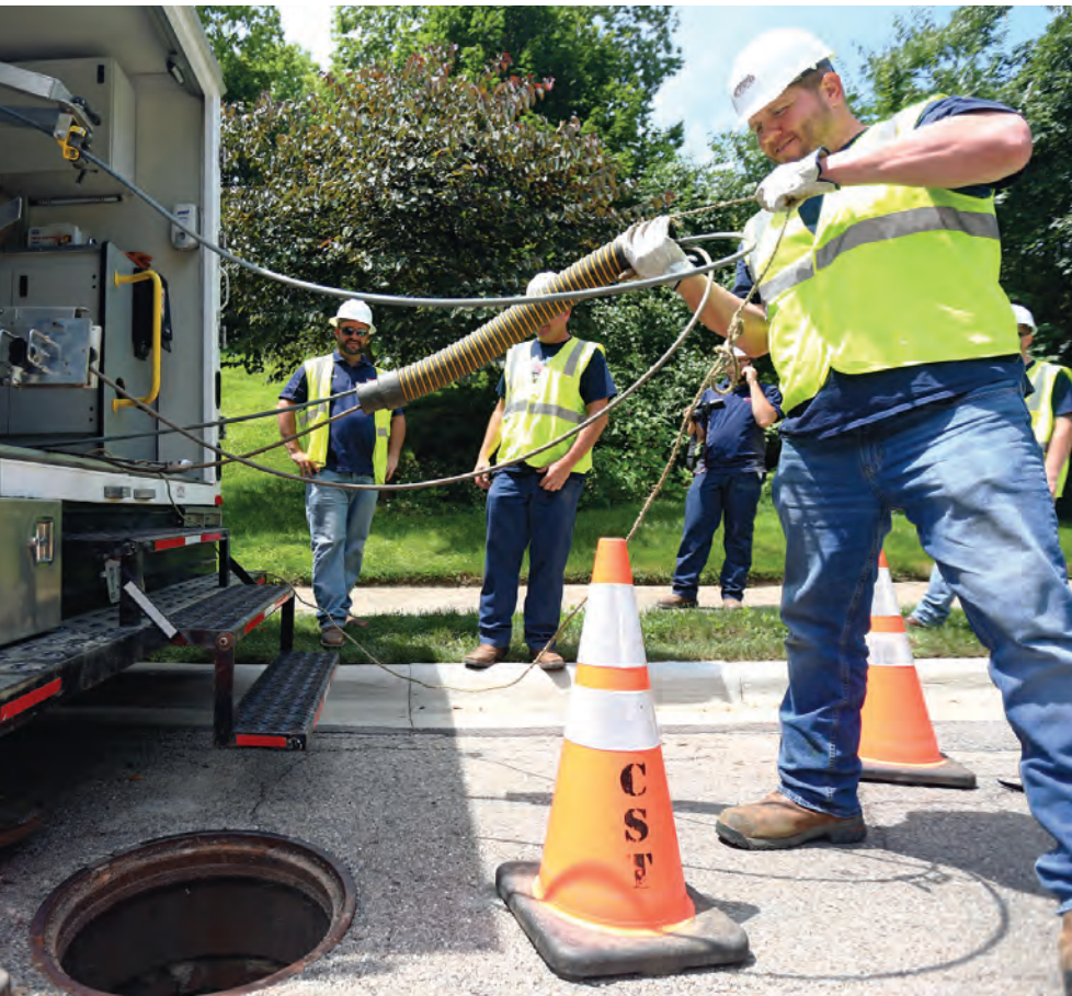
Bucky Skaggs (right) sets up for a sewer main inspection in Columbus, Ohio.
