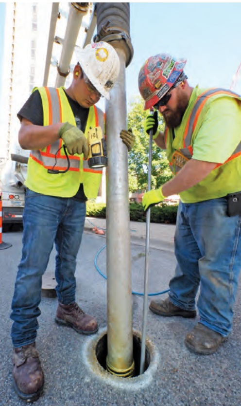
Davids Hydro Vac laborer Jason Bauer (left) and operator John Shuneman clean out a utility access point along a street in downtown Minneapolis.
