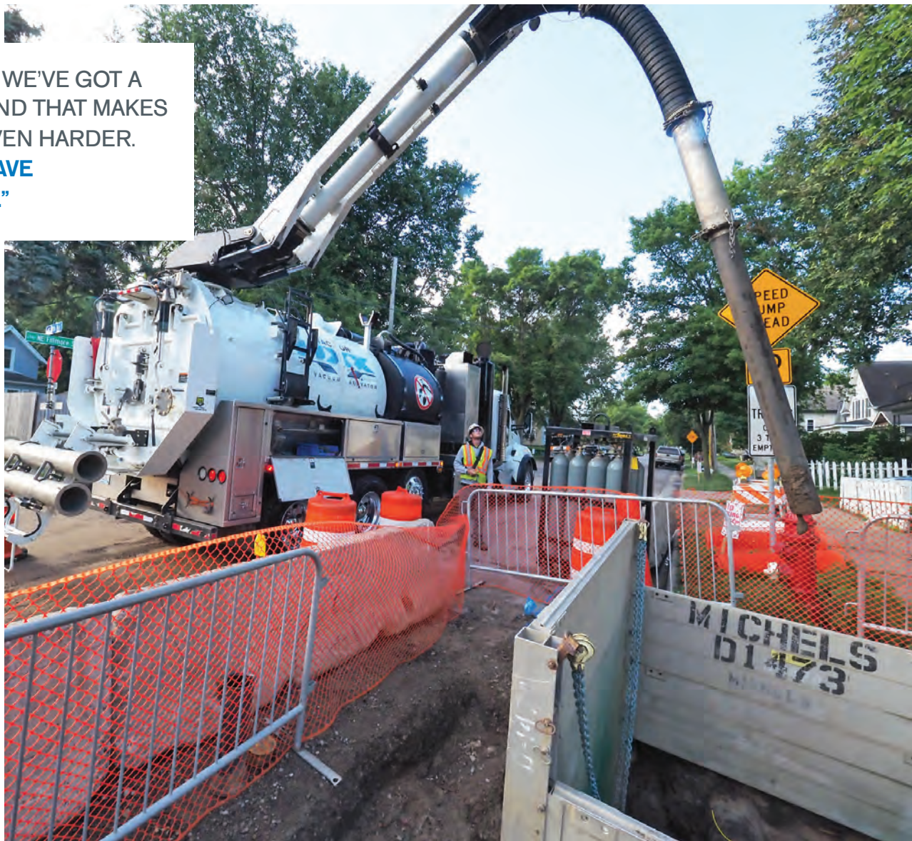
Randy Becker guides the Vector HXX hydroexcavator’s boom inside a shored trench while he and laborer Nate Otto clear the site for a utilities relocation project.
