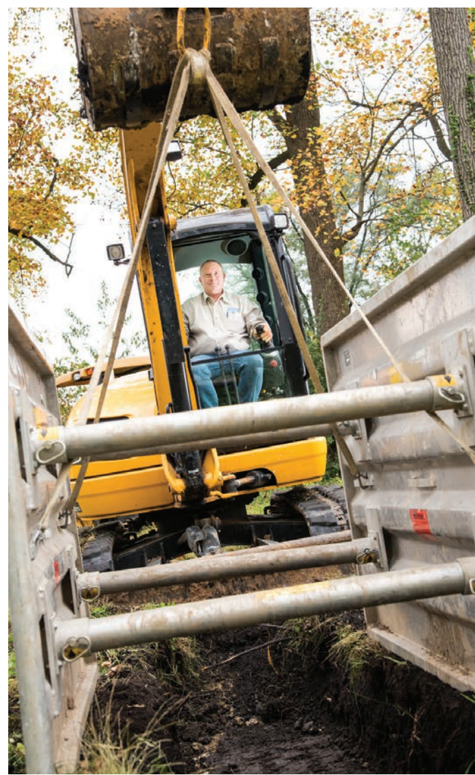
BELOW Shawn Berroyer positions an Ultra Shore trench box for a residential sewer repair.
