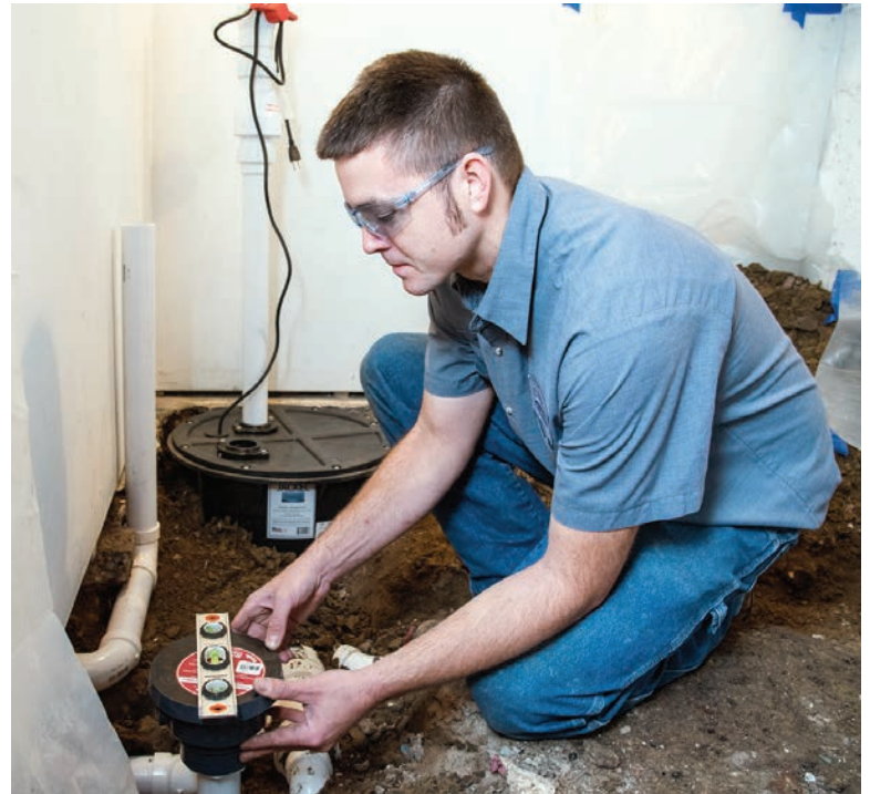
BELOW Jimmy Walters adjusts a Sioux Chief FinishLine and floor drain that is hooked to a Jackal sewage ejection pit.
