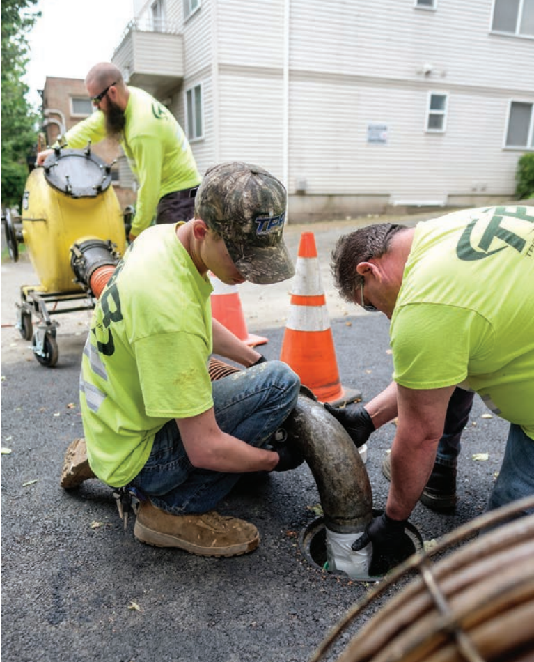
A crew shoots a liner into a residential sewer lateral from a cleanout in the driveway.
