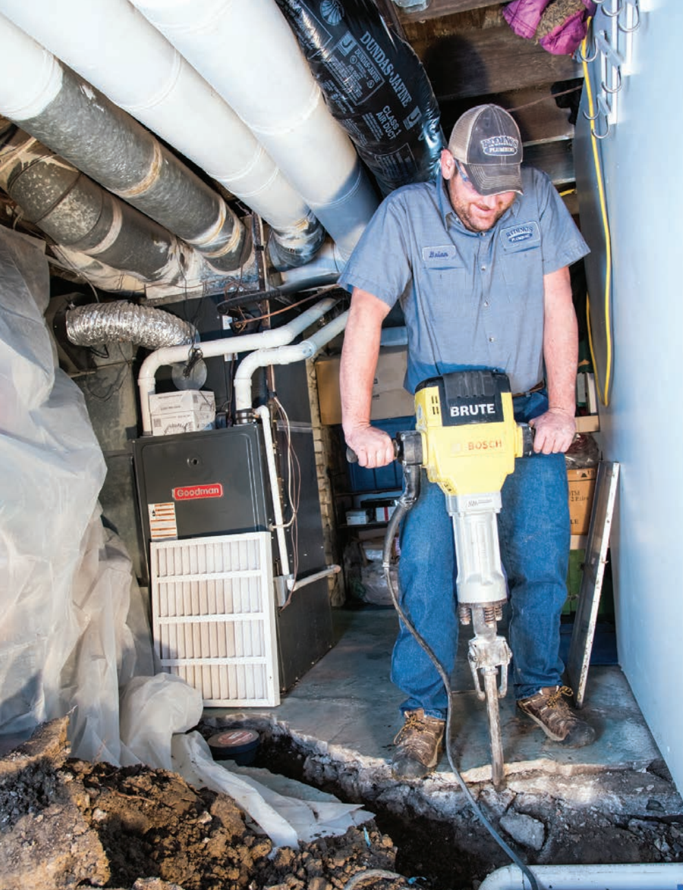
<< Brian Holmes uses a Bosch Breaker Hammer to open up a basement slab and begin reconfiguring the home's drain system. The job is part of a city of Springfield program to minimize basement backups.
