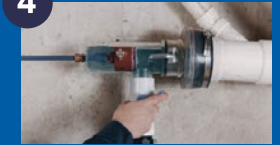
OPEN VALVE AND DRAIN CONTENTS
