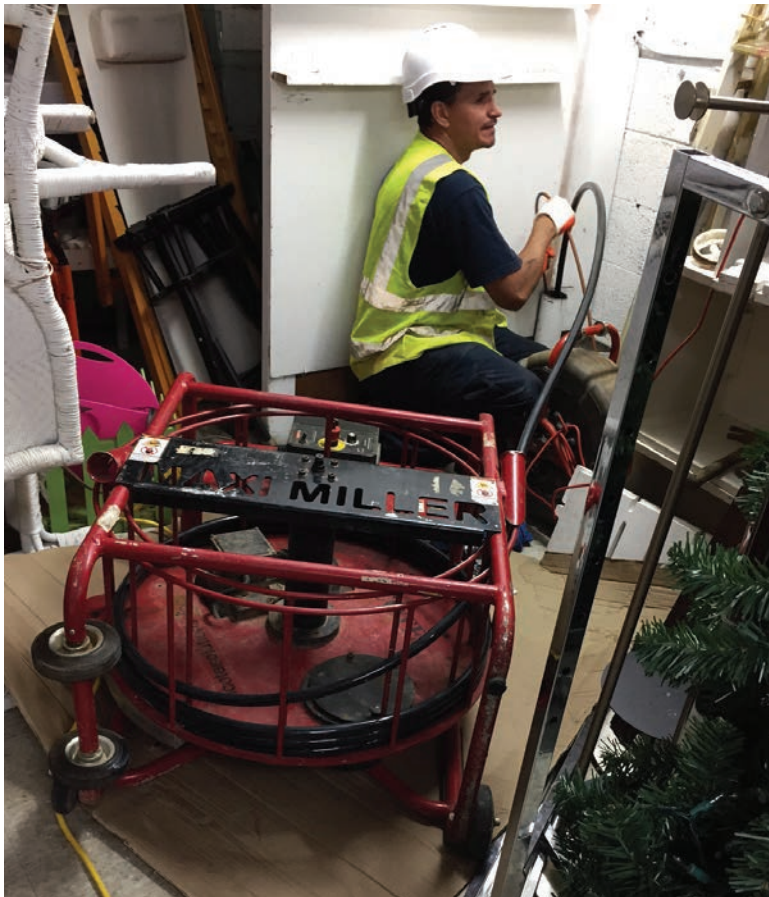
Nehemiah Martinez of All American Plumbers uses a Maxi Miller from Picote Solutions to descale a 4-inch-diameter cast-iron sewer line at a commercial shopping center.
