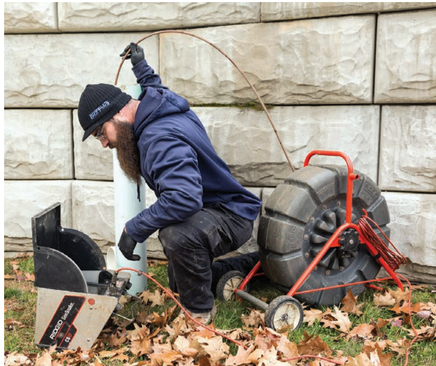
Keeping your hands near the drain opening and feeding the camera into the line slowly will help prevent kinking the reel and damaging your push camera.
