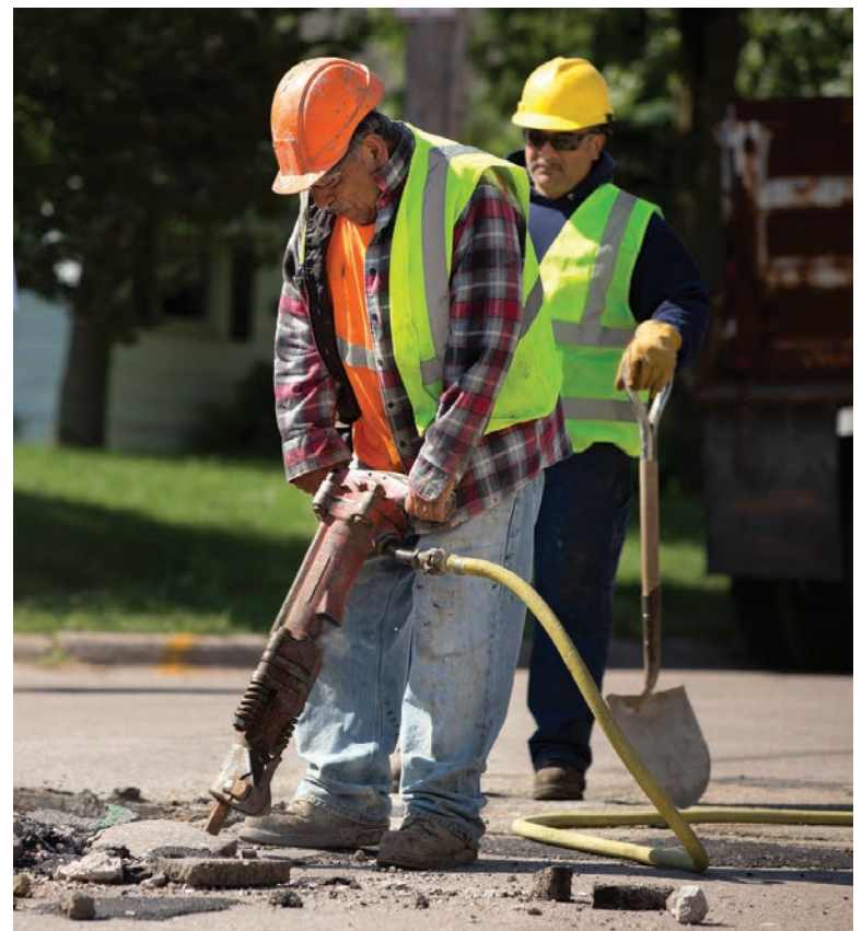
Roberto Lopez jackhammers surface material around a manhole at the start of a rehabilitation project in Davenport, Iowa.
