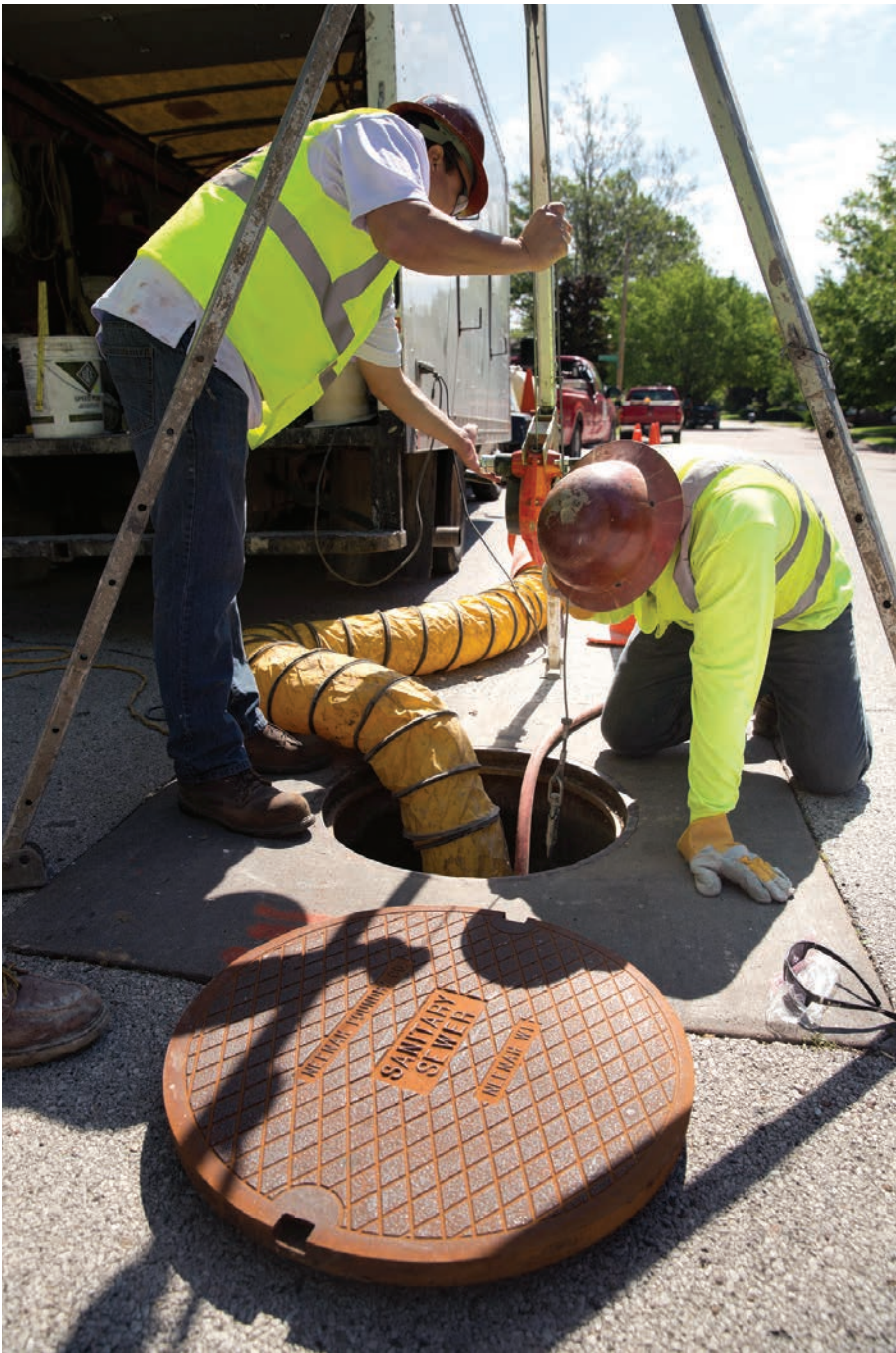
◀◀ Brett Vallow (left) and foreman Mike Walsh visually inspect a cement liner, measuring vertical footage for build quantity.
