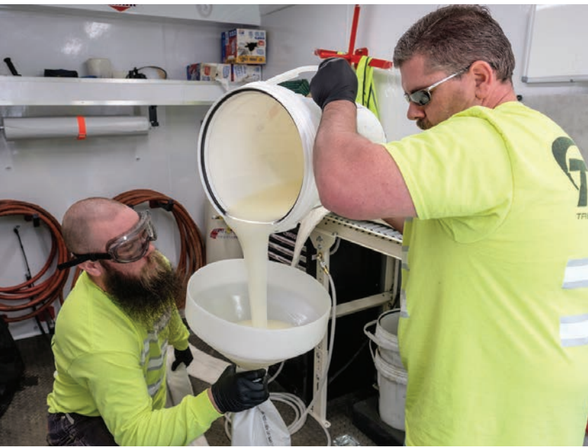
ABOVE Mike Wasmund pours resin into a liner held by James Tryon in preparation for a CIPP repair.
