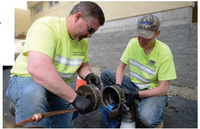
<< James Tryon controls air pressure at the Perma-Liner inversion unit while Mike Wasmund and Eric Poteet install a CIPP liner in a municipal sewer line.
