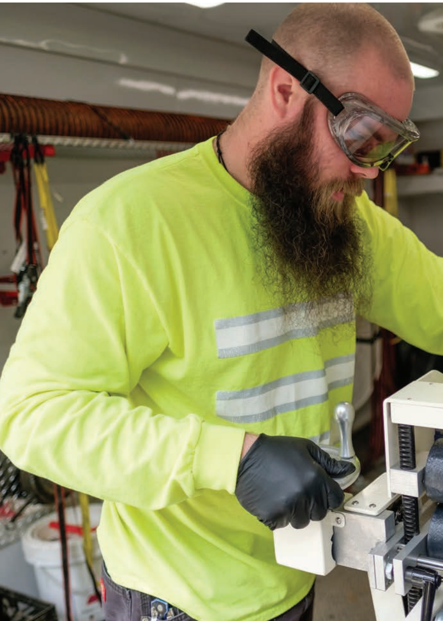
BELOW Tryon, Wasmund and Poteet (from left) feed a liner through the roller to impregnate it with resin prior to installation.
