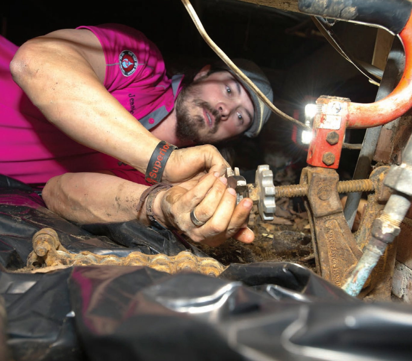
<< LEFT Jessie Wigley cuts through a leaking cast iron pipe under a house.
