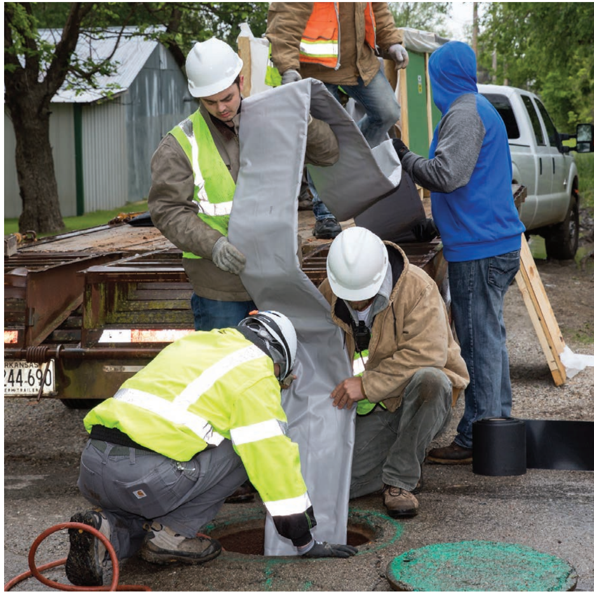
LMK Technologies' Schwalm Robot operator Kyle Mucci (center) helps unload an ultraviolet liner while Saertex-multiCom sales representative Tim Lupia (left) and Humbard Contracting laborer Malcolm Brumley guide the liner into a manhole.
