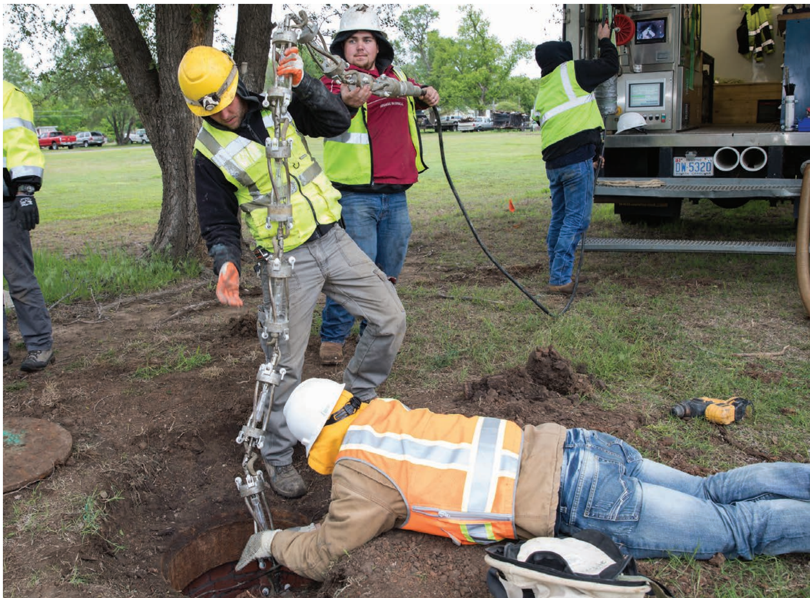
ABOVE Saertex-multiCom lead technician Alex Kaefer (left) lowers the ProKASRO light train into the manhole as project superintendent Quinton Humbarb (center) and laborer Cody Kilgore assist on a lining job in Blackwell, Oklahoma.
