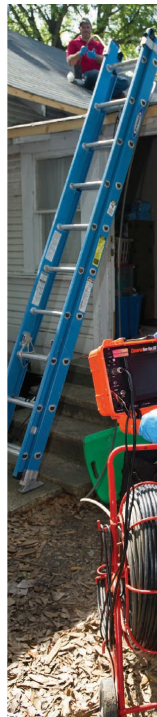
BELOW Jessie Wigley watches the monitor on a General Gen-Eye SD inspection system while Andrew Horton feeds the camera down a vent stack from the roof.
