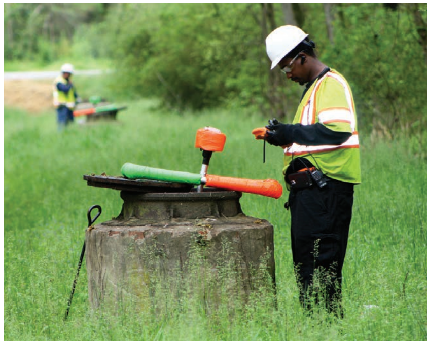
Brandon Smith (foreground) and Exavier Moceton of Ace Pipe Cleaning make a quick assessment of a sewer line segment with the SL-RAT.
