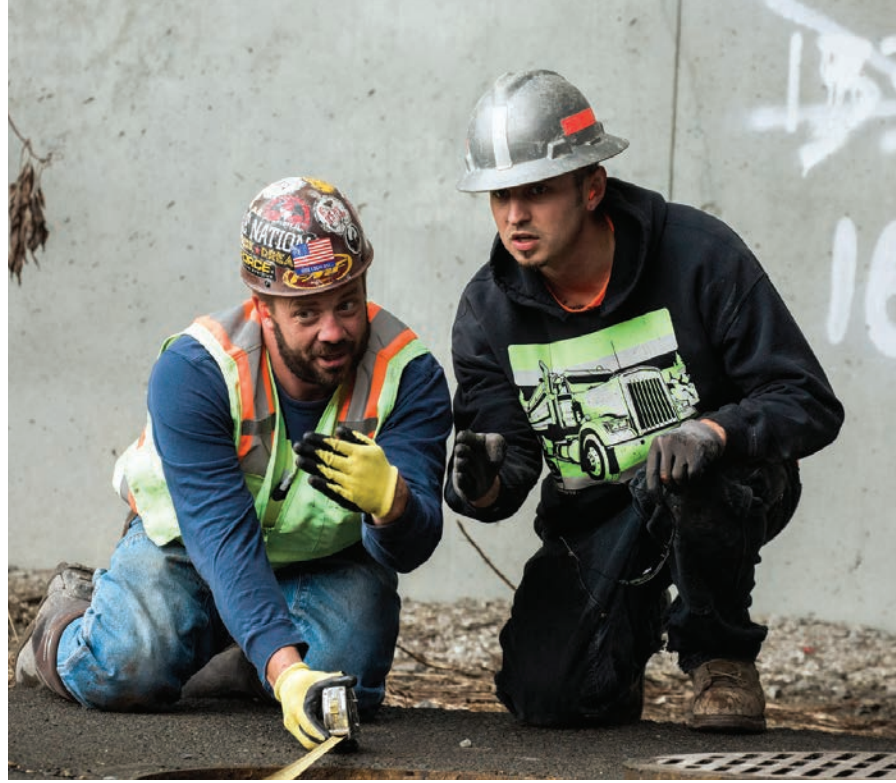
Brian Minter (left) and John Raring estimate the location of a pipe at the Port of Tacoma.
