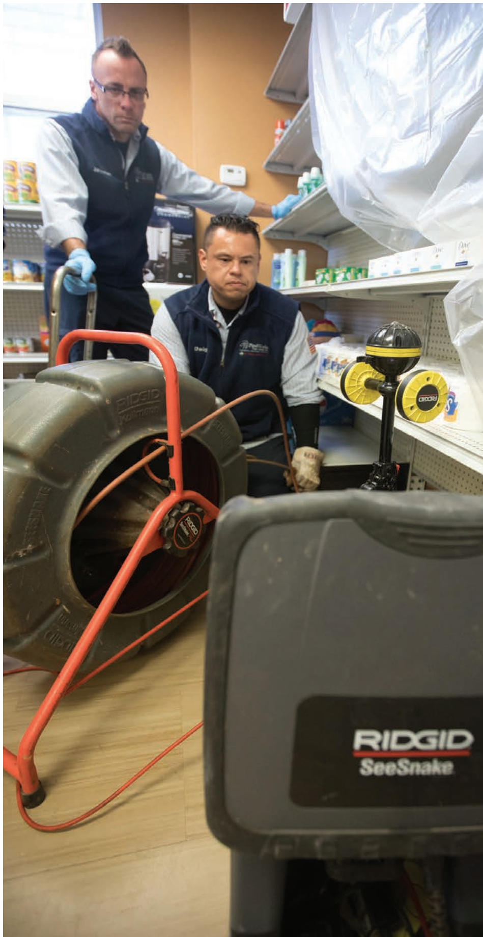
Technician Dwight Rodriguez feeds a RIDGID SeeSnake into a clean-out to find the source of a blockage, while senior technician Jonathan Dorieux looks on.
