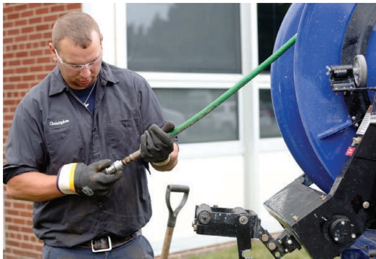
Mike Justus switches jetting nozzles before cleaning a sewer line at St. John's School in Ashtabula.
