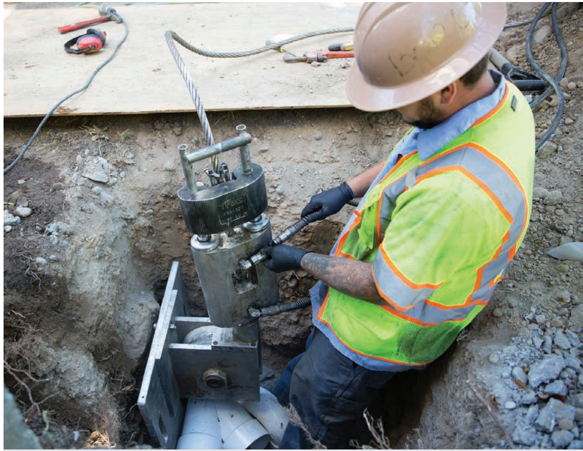
Josh Lemrey sets up a TRIC Tools pipe bursting machine to replace a concrete sewer line.
