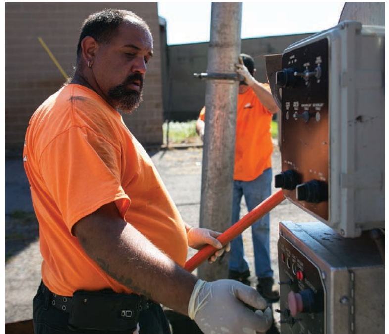
Cain Catino keeps his hand on the controls of a Vactor 2100 while cleaning a sewer line with Charles Castrechino.
