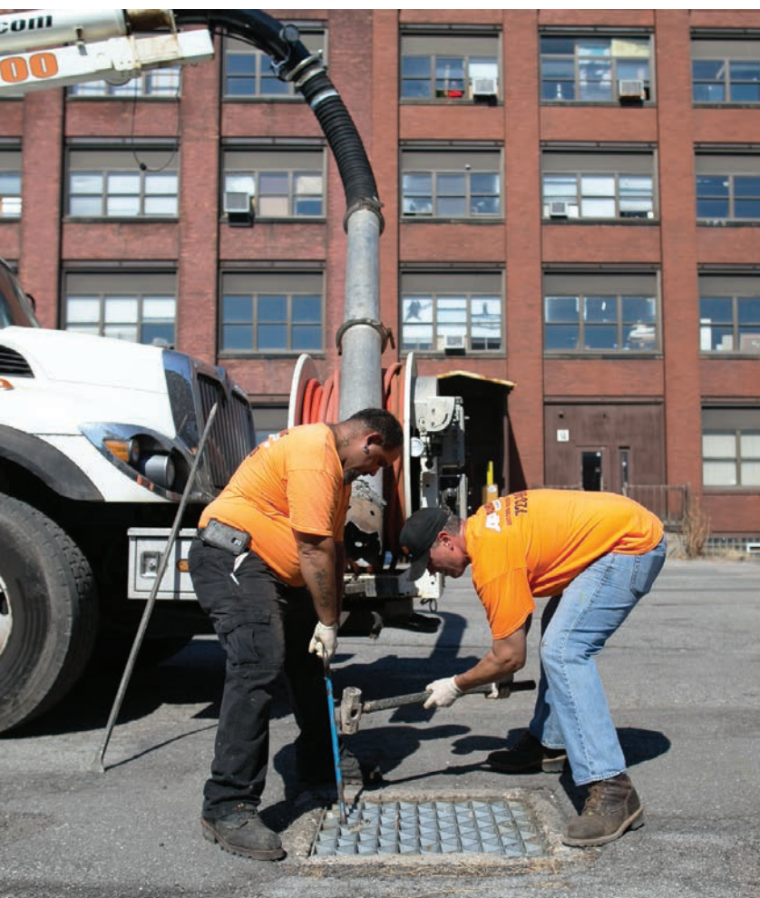
Commercial technician Cain Catino (left) and industrial technician Charles Castrechino of AP Plumbing lift the lid on a drainline outside an industrial facility in Rochester, New York.
