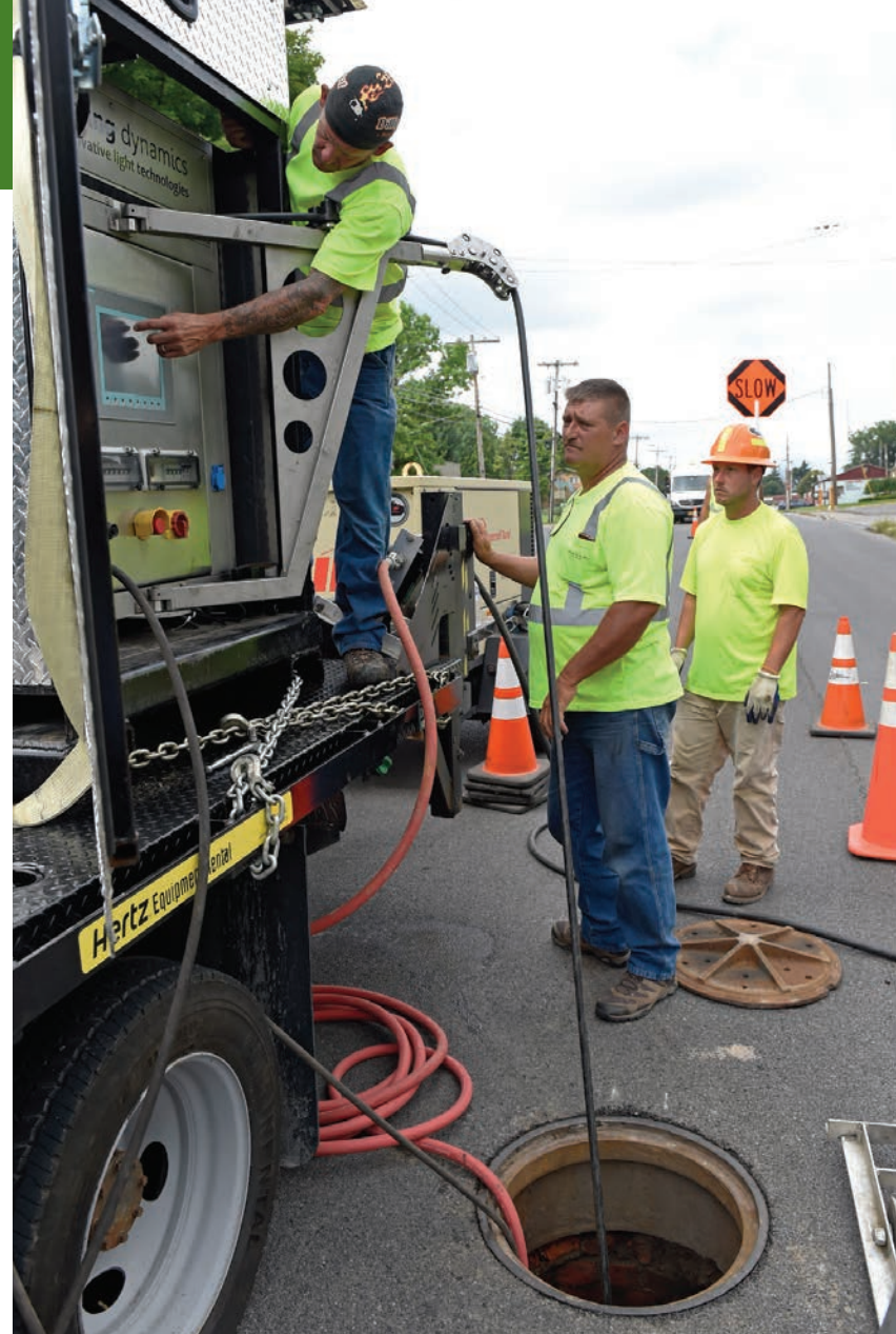
Precision Trenchless UV operator Mark Witthohn reaches for the UV light train control panel to power down the unit after curing a fresh liner in a 10-inch-diameter sewer line. Field supervisor Tim Nappi (center) and cutting camera supervisor Robert Chrysler were also working on the project.
