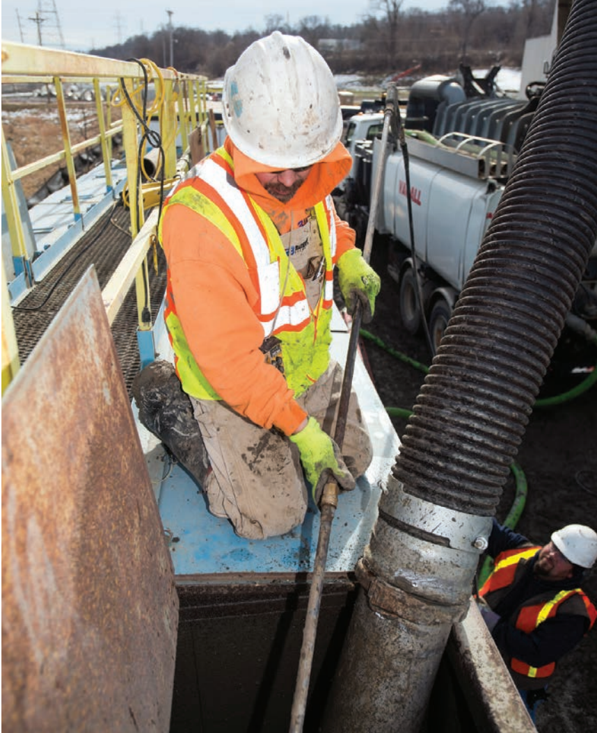
Jamey Severn uses a pressure washer connected to a Vacall hydroexcavator to loosen sediment from a dewatering tank.
