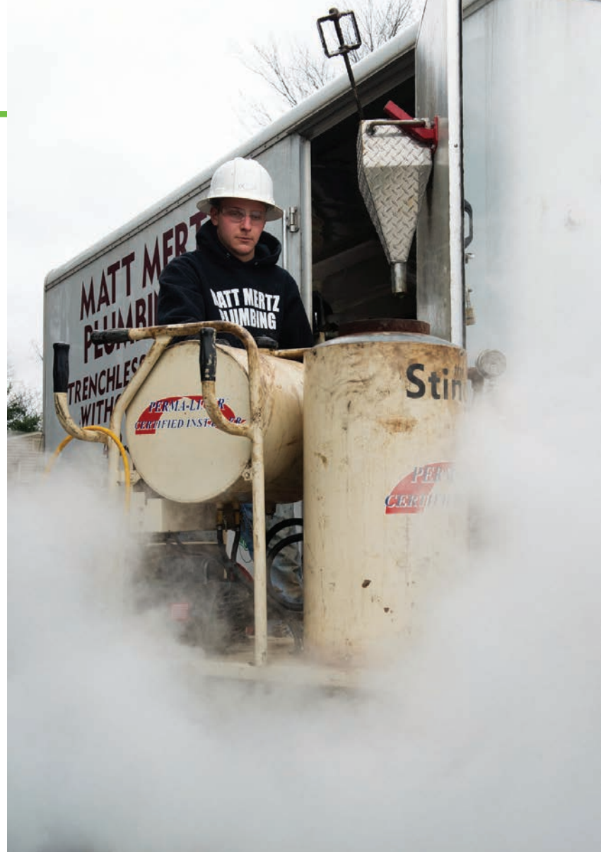
Dylan Belfiore, a plumber with Matt Mertz Plumbing in Pittsburgh, Pennsylvania, runs a Perma-Liner Stinger mini steam unit during the installation of a residential lateral liner.
