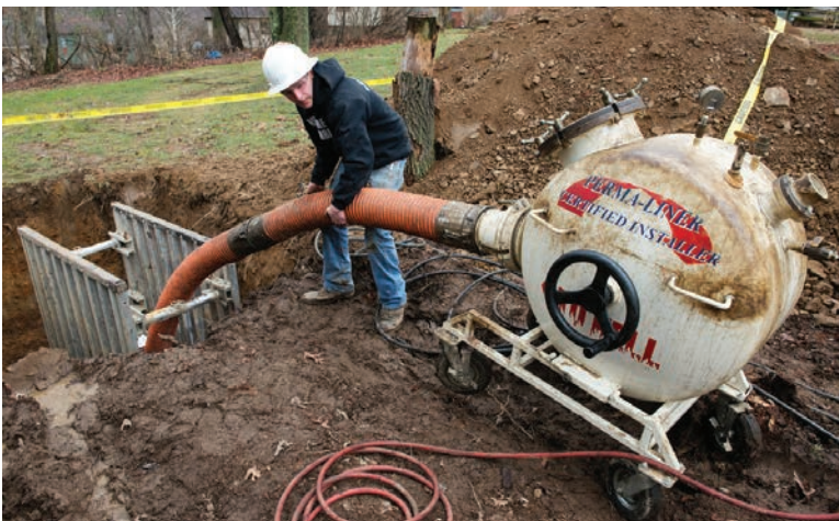
Dylan Belfiore guides the Perma-Lateral inversion unit (Perma-Liner) at the entry pit on a lateral relining job.
