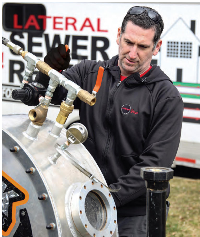
Liner Guys co-owner Mike Rodger monitors the air pressure on an LMK lateral inversion tank while lining a residential sewer lateral.
