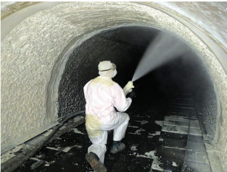
A member of the J.R. Pipeline crew sprays structural polymer on the clean pipe interior.
