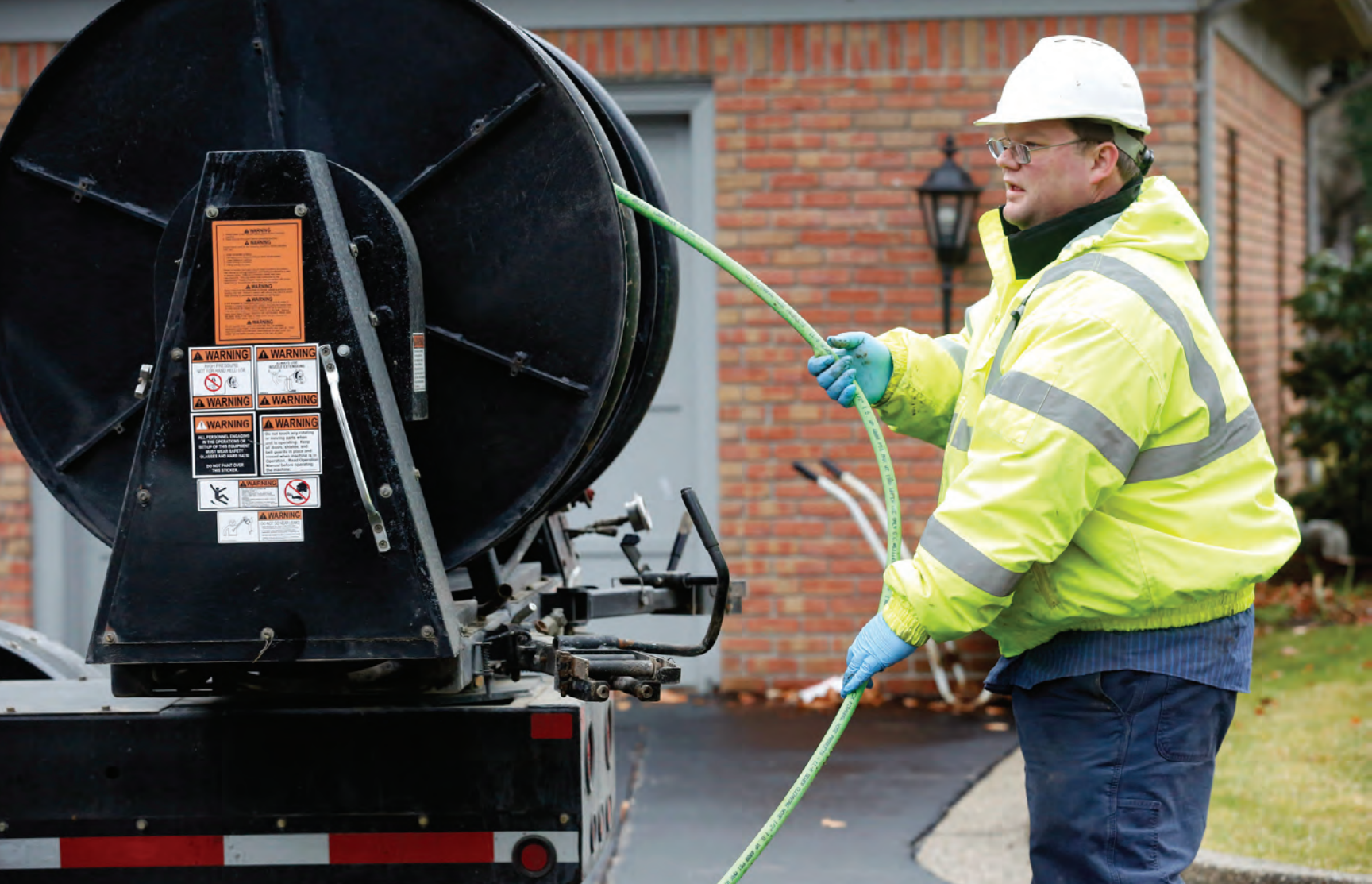
Jim Simpson unspools hose from a trailer-mounted Sewer Equipment jetter while setting up for a cleaning job in Grosse Pointe, Michigan.
