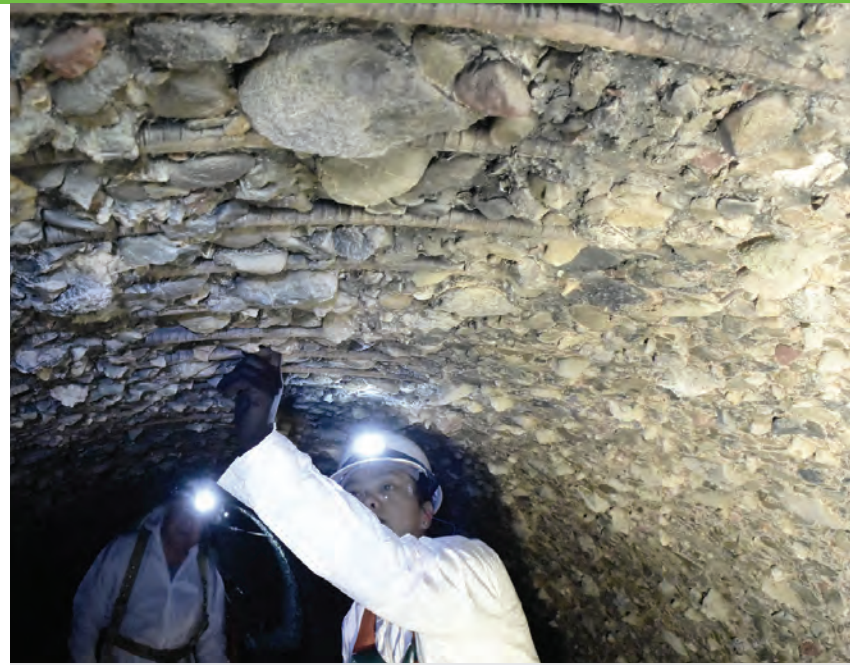
Hydroblasting the interior of the East Bay Municipal Utility District's 75-year-old Wood Street Interceptor removed old mortar and exposed river rocks, creating a bumpy surface that made lining difficult.
