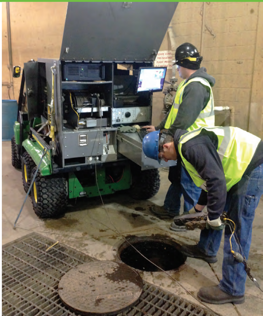
Hydro-Klean operator Hans Nissen gets ready to launch the camera while foreman Zack Myers handles the controls of the CUBE portable mainline inspection system from R.S. Technical Services. The CUBE system allows Hydro-Klean employees to inspect sewer lines in remote and limited-space situations.
