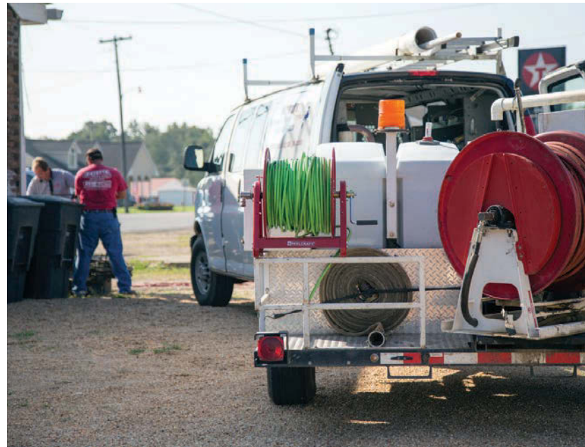
Fayette Drain & Sewer's trailer jetter from US Jetting provides extra muscle on tough drain cleaning jobs.
