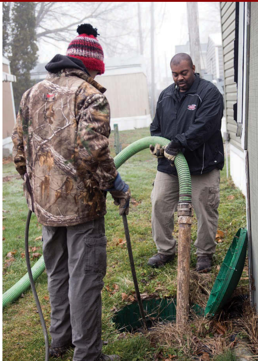
Cooper Wallace (left) jacks a septic tank while Floyd Griffin pumps it out. Sewer and septic systems in local trailer parks have provided a good source of business for All Around Pumping.
