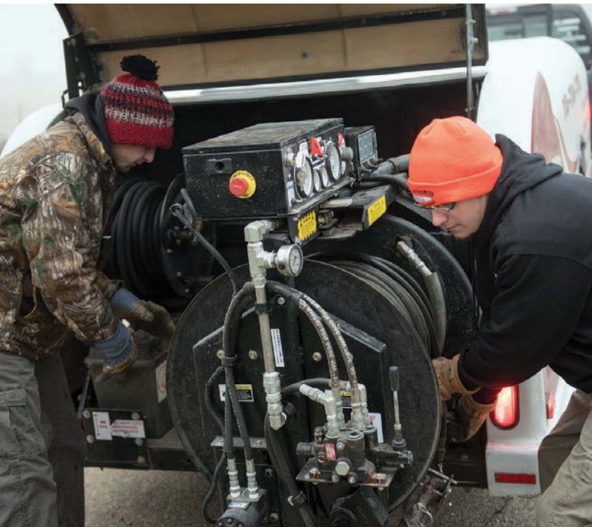
Cooper Wallace (left) and Cody Hinrichs set up the enclosed Spartan trailer jetter before cleaning a septic tank.
