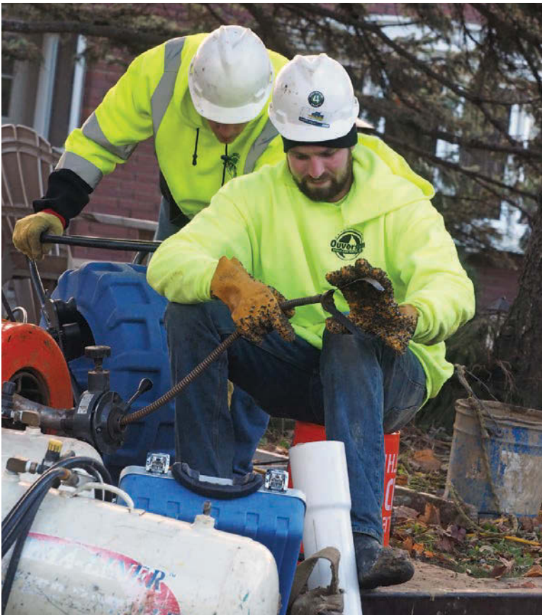
Technicians David Allen (left) and Matt Allen set up for the preliminary cleaning and inspection of a lateral line before repairing it with CIPP.
