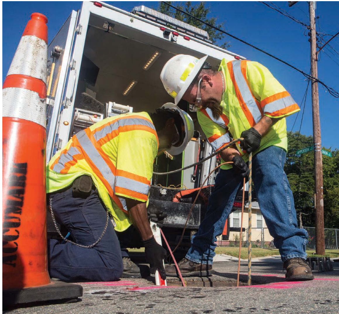
Robert Wilson (left) and Bryan Reese maneuver an inspection camera into a raised sewer line along Union Street in Richmond, Virginia.
