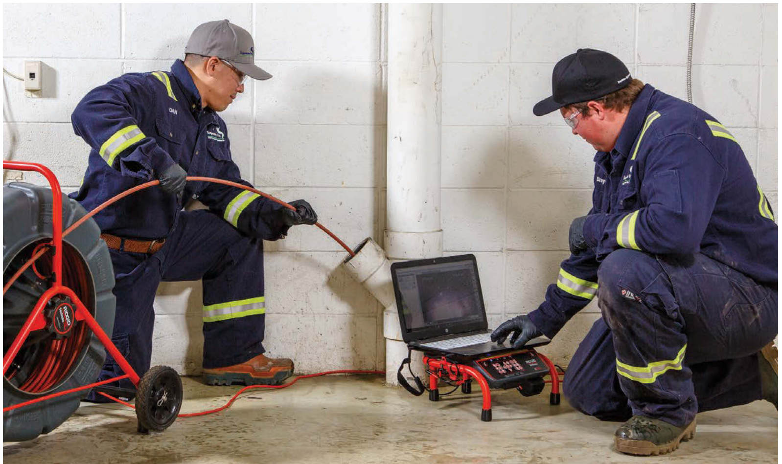
Dan Lin (left) and Braydon Jeske inspect a drainline with a RIDGID SeeSnake Plus.
