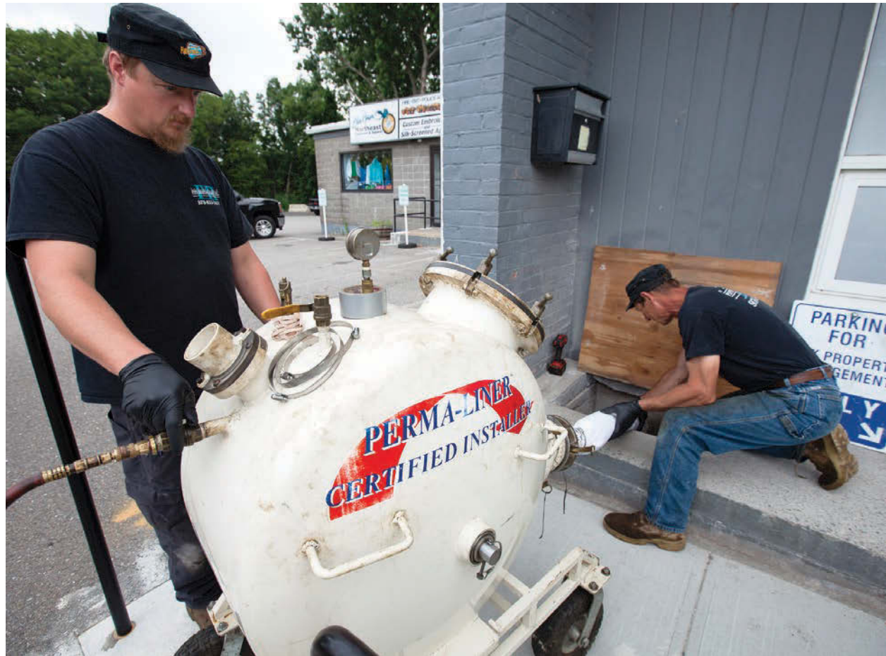
Matt Leger (left) operates a Perma-Liner Perma-Lateral inversion unit while Frank Machonis helps feed the liner into the pipe.
