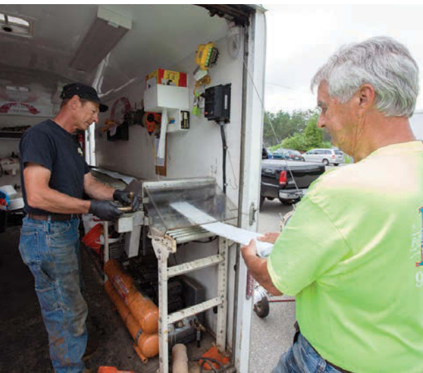
ABOVE: Bernie Tessier (right) helps move a liner into position as Frank Machonis begins the wet-out process.
