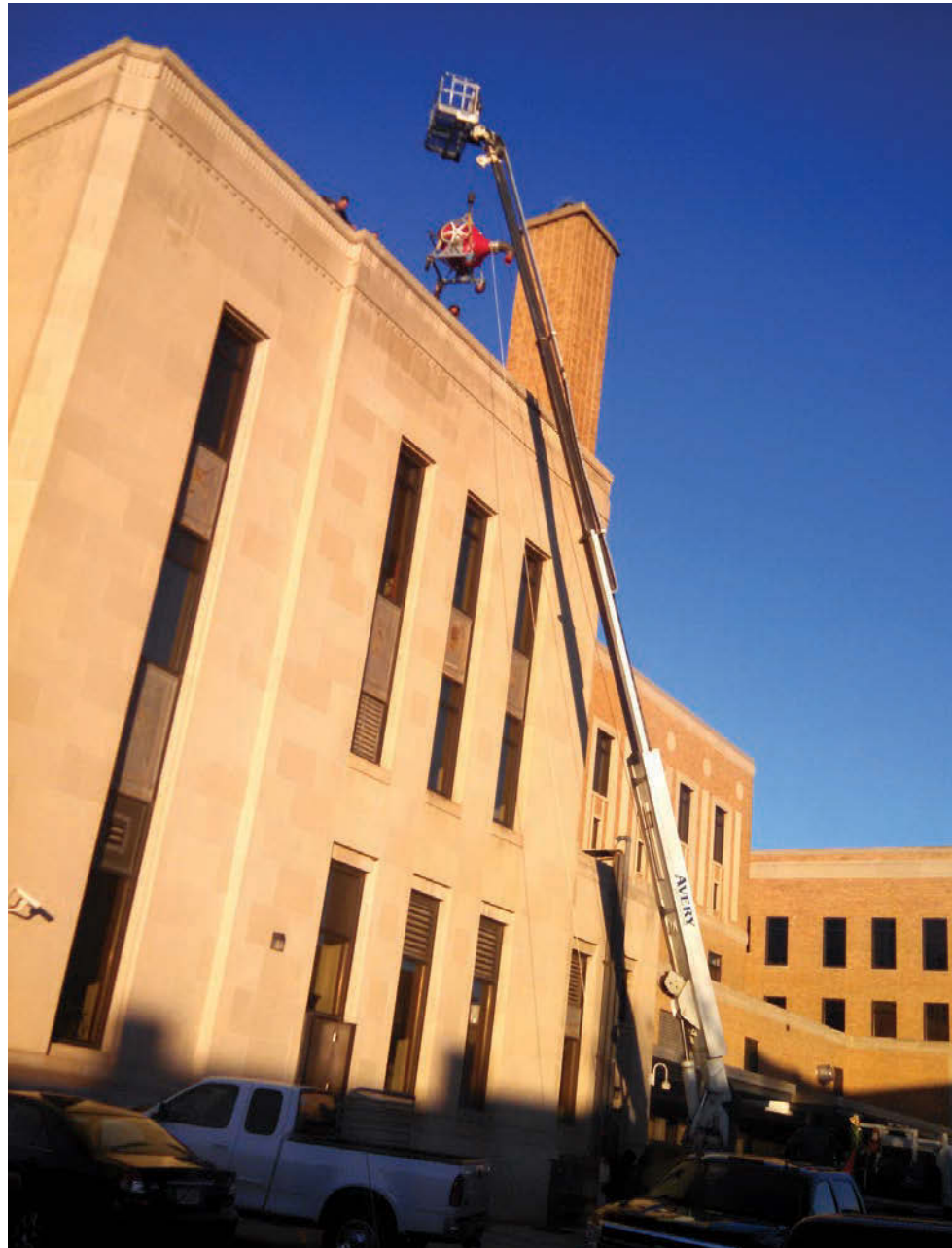
Equipment is lifted to the roof of the historic federal building and U.S. District Courthouse in Sioux City, Iowa, for a stormwater drainage system rehabilitation project.
