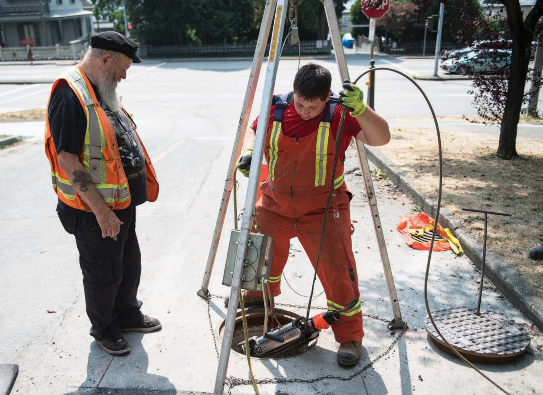
Devlin Hawkes of ABC Pipe Cleaning Services lowers a CUES Shorty CCTV camera into a manhole for a sewer main inspection in New Westminster, British Columbia.
