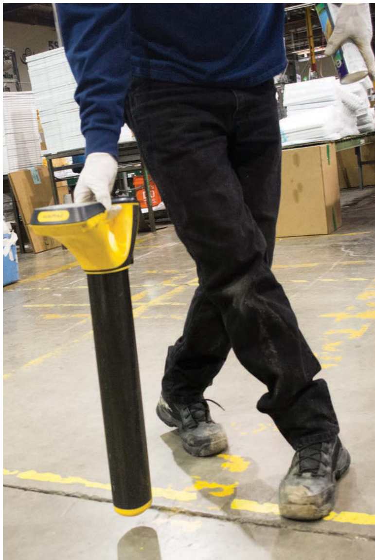
Larry Stegmaier uses a Vivax-Metrotech vLocCam 2 locator to pinpoint the location of a problem in a commercial building.
