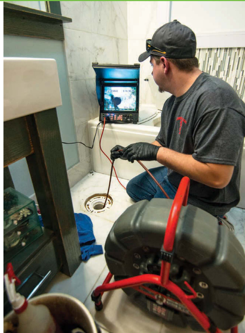
Sewer Duck technician Jeremy Sitter inspects a bathroom drainline with a RIDGID SeeSnake pipeline inspection system.
