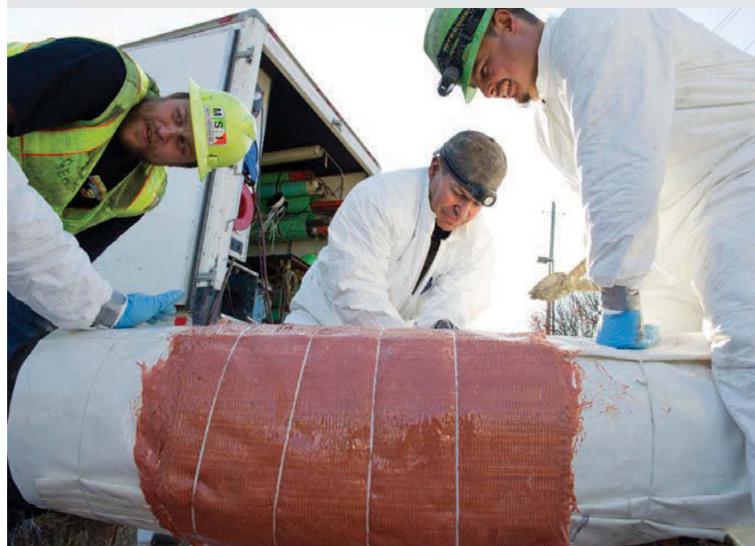
BELOW: Miksis crew members (from left) Geoff Ensign, TJ Sales and Ben Robles roll a polyresin-coated fiberglass liner onto an inflatable plug for a point repair.
