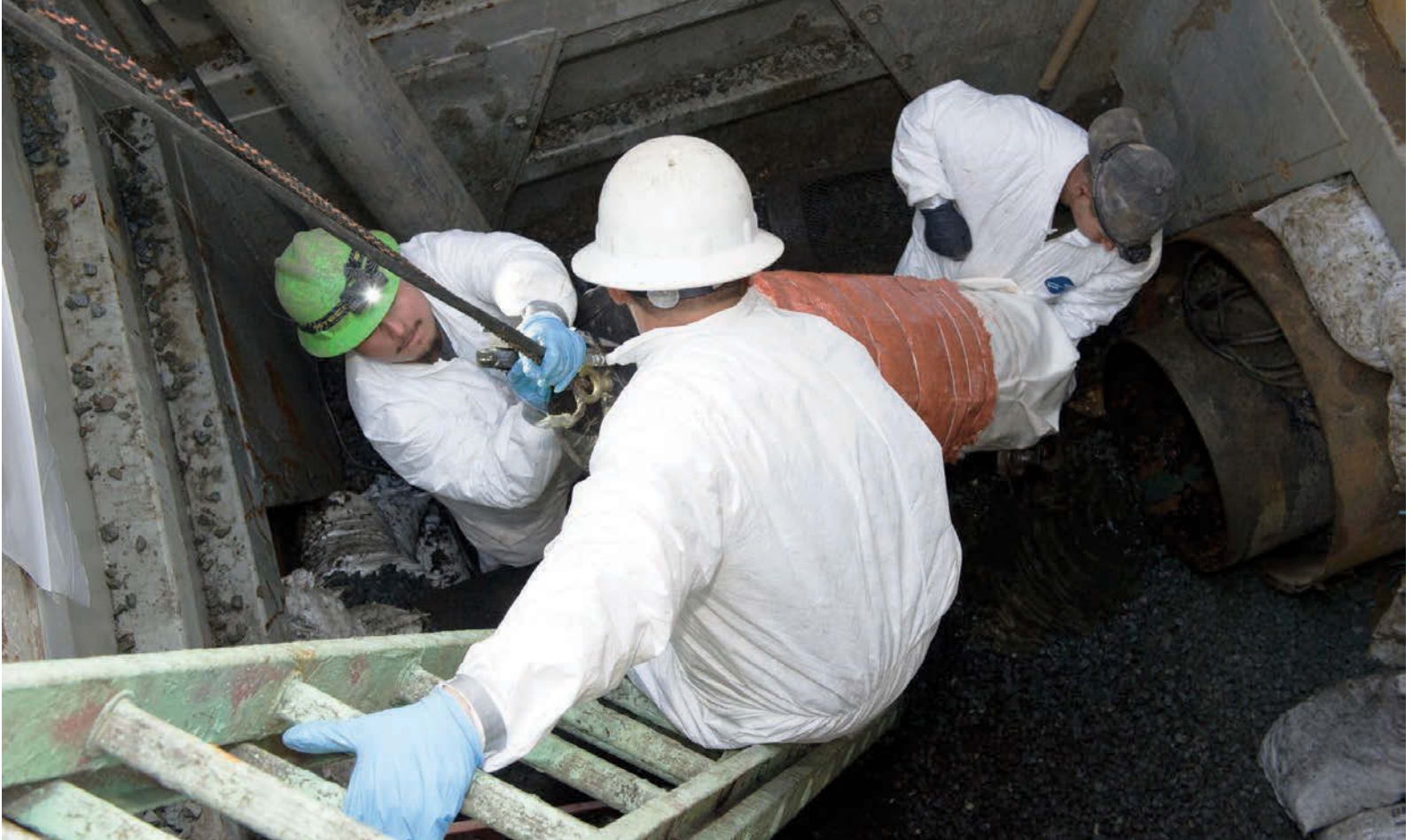
Miksis Services workers (from left) Ben Robles, Manuel Lemos and TJ Sales insert an inflatable carrier with a polyresin-coated fiberglass composite point repair liner into a 24-inch water main.
