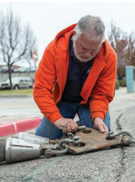
Jay Garrett sets up the triangular steel plate for a double pull. For this triple-burst job, he designed a different 1.5-inch-thick steel plate with three holes for mounting pipe and a center hole for bolting it to the burst cone.
