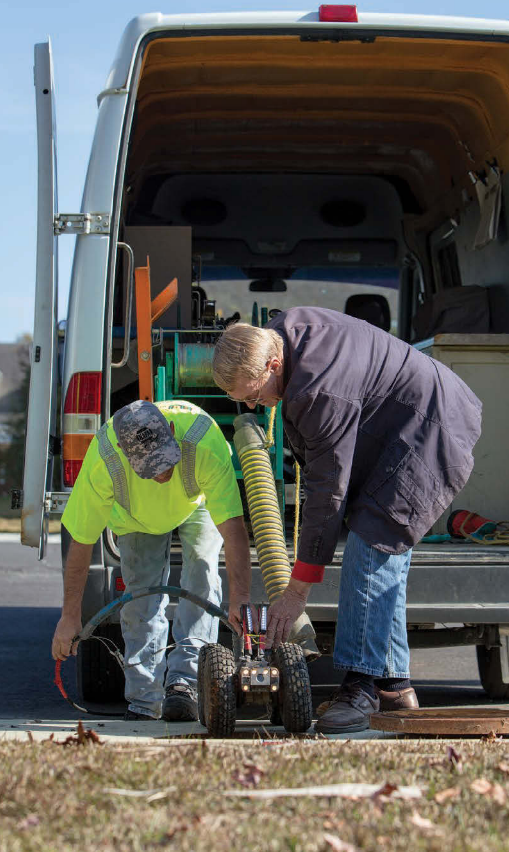
John May (right) and camera operator Richard Begnaud retrieve the Cyclops inspection camera from a manhole after inspecting a pipe segment.
