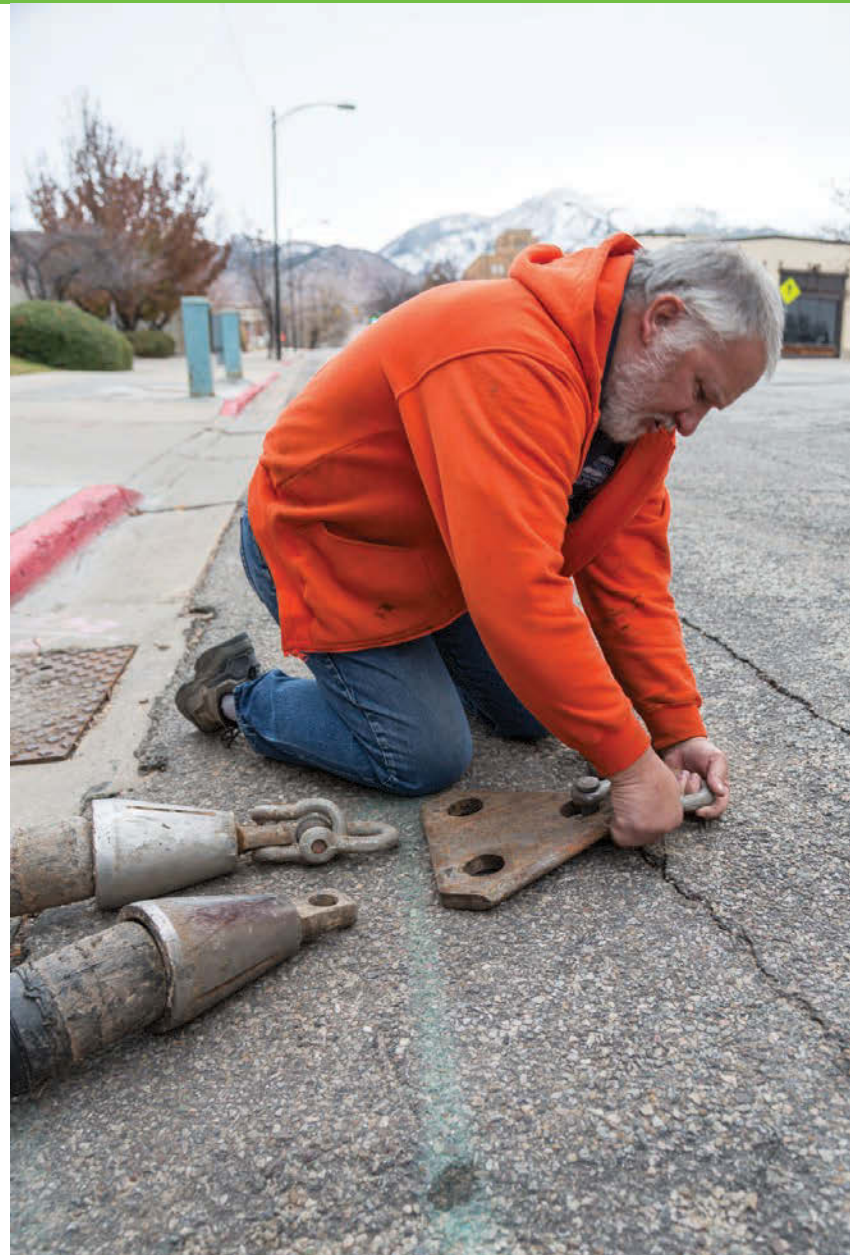
Utah Pipebursting owner Jay Garrett attaches two HDPE pipes and the swaged cable to the triangular steel plate he developed for replacing dual laterals simultaneously.
